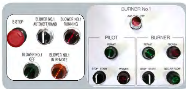
Cooling air blower and igniter burner controls.
