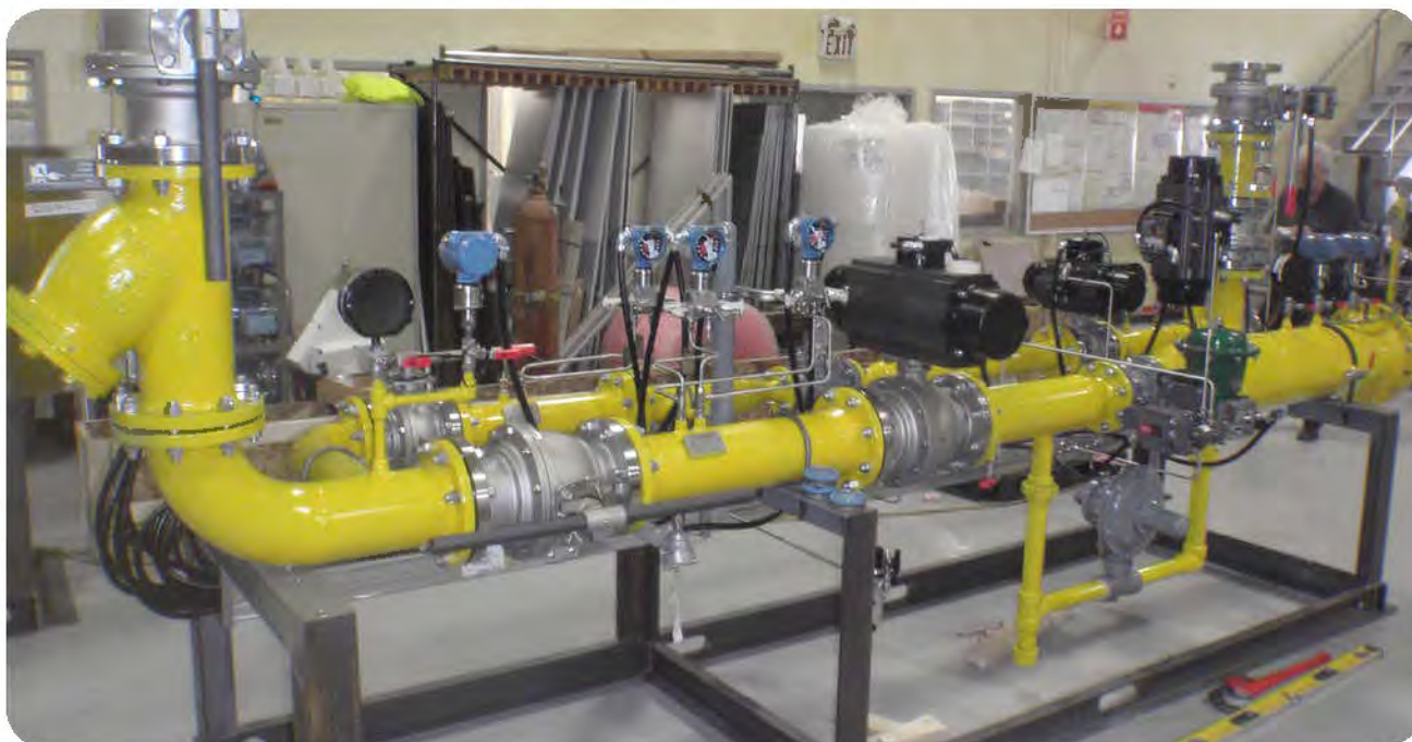
Shop-assembled main gas header valve train.
