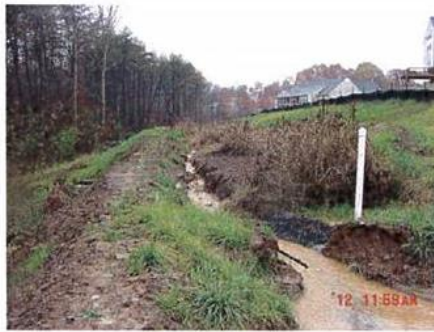
Bioretention swale, installed too early during active construction, has become clogged with sediment.
