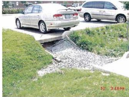
Curb inlets to bioretention swale have eroded because of improper sizing of stone.
