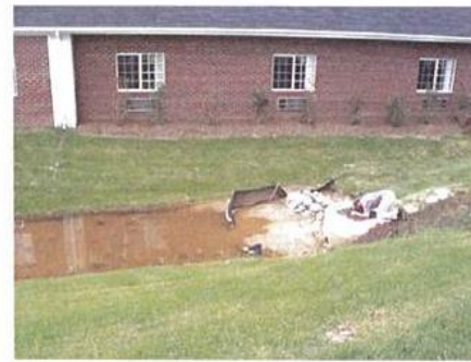
Bioretention area does not drain because of improper soil media, soils compacted during installation, and/or filter fabric under media.
