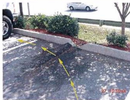
Site runoff by-passes bioretention swale because of small elevation changes during construction.
