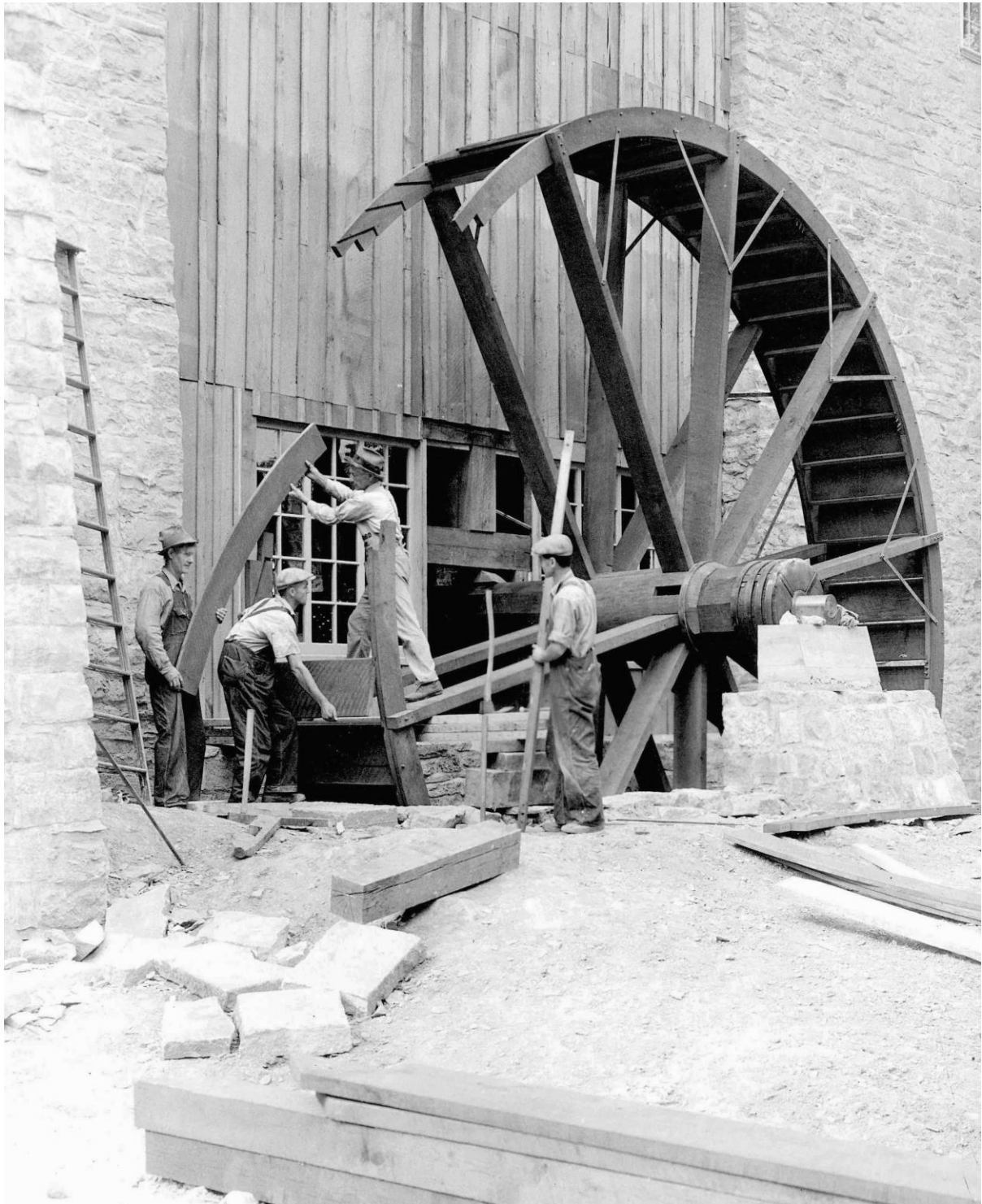
Spring Mill Waterwheel Construction, 1930, photo by Denzil Doggett, in Water-Powered Mills Committee Collection , Indiana Historical Society
