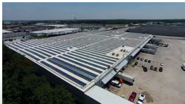
Grocers Supply Roof, 1MW rooftop system.
