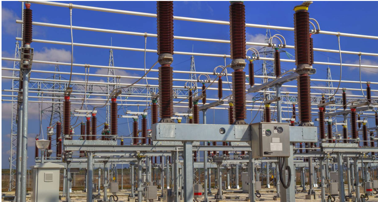
Figure 13: Substation Circuit Breakers are Used to Change System Topology.
