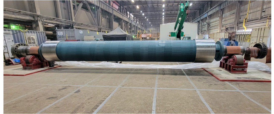
Gibson Unit 3 Generator Rotor
