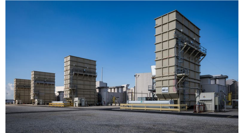
Wheatland Generating Station
