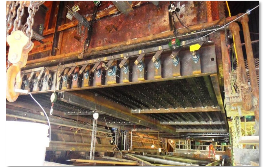
Gibson Unit 1 Boiler Backpass Dampers
