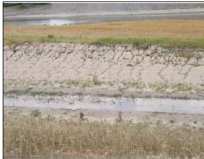
Figure 5.23-2: Typical Construction Site Erosion
