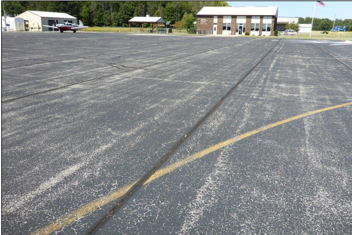
Figure 2-5. Typical AC Pavement in Fair Condition (Feature 3010)
