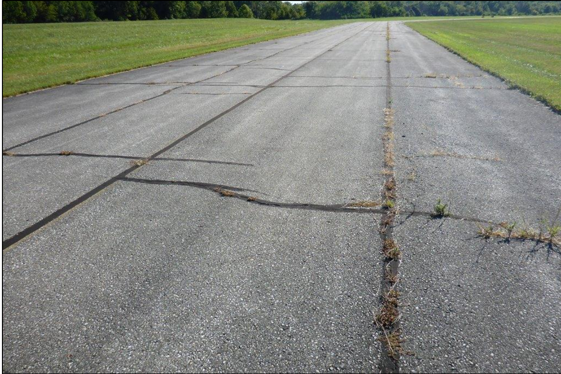
Figure 2-6. Typical AC Pavement in Poor Condition (Feature 105)
