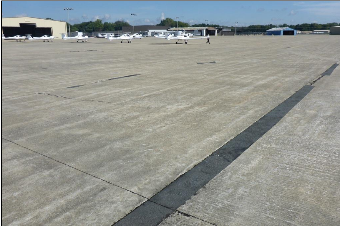
Figure 2-5. Typical PCC Pavement in Poor Condition (Feature 3001)
