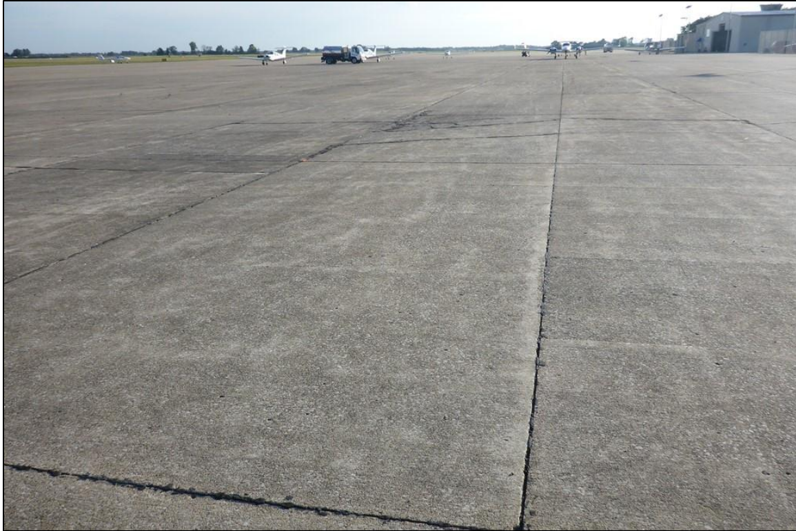
Figure 2-4. Typical PCC Pavement in Fair Condition (Feature 3002)
