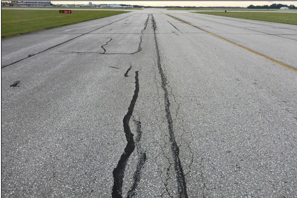
Figure 2-7. Typical AC Pavement in Poor Condition (Feature 202)
