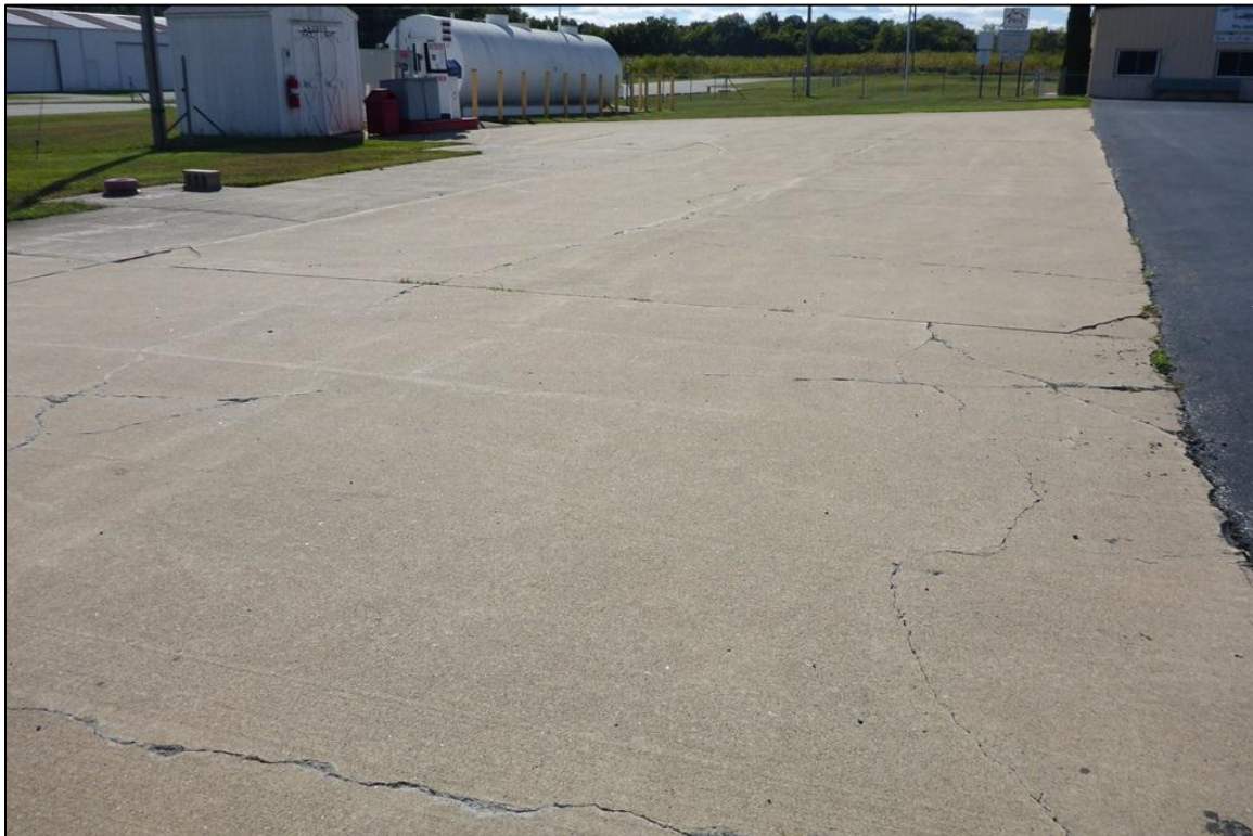
Figure 2-3. Typical PCC Pavement in Poor Condition (Feature 3005)
