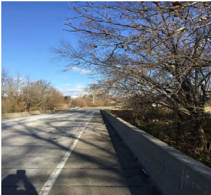
PHOTO 1 Description Trees growing over East side of bridge
