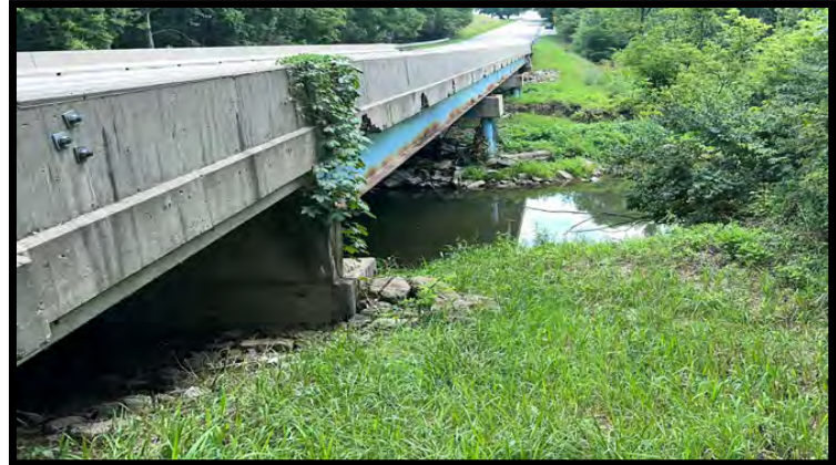
Photo 60: Looking southeast along the west side of the bridge from the northwest bank of Big Blue River.
