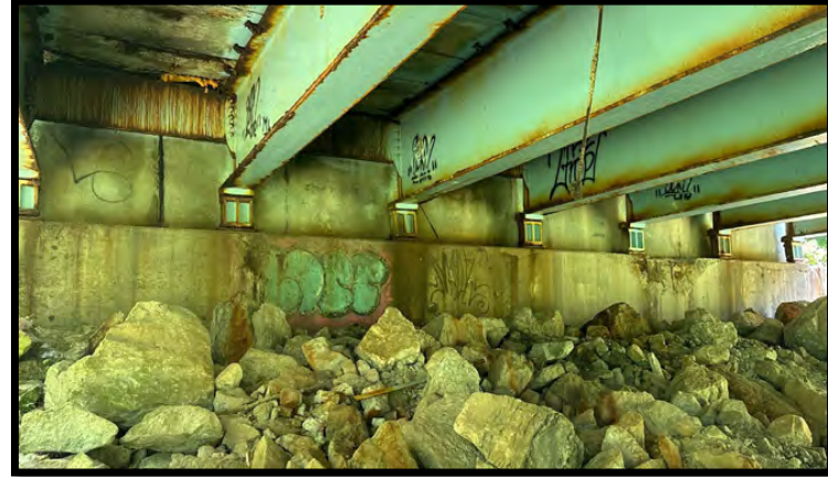
Photo 50: Looking southeast at the south headwall of the bridge. There were no signs or bats or birds.
