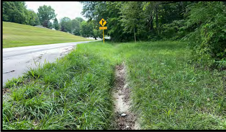
Photo 37: Looking southeast at the beginning of RSD3, from the southwest corner of the investigated area.
