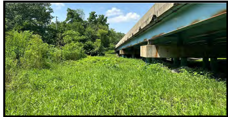
Photo 48: Looking northwest at the grassy area along the southwest side of the bridge.
