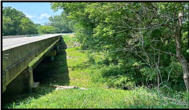
Photo 23: Looking northwest along the bridge from the southeast corner of the bridge.
