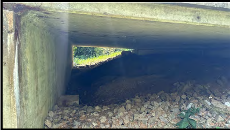
Photo 59: Looking northeast through the north end of the bridge. There were no signs of bat or birds.
