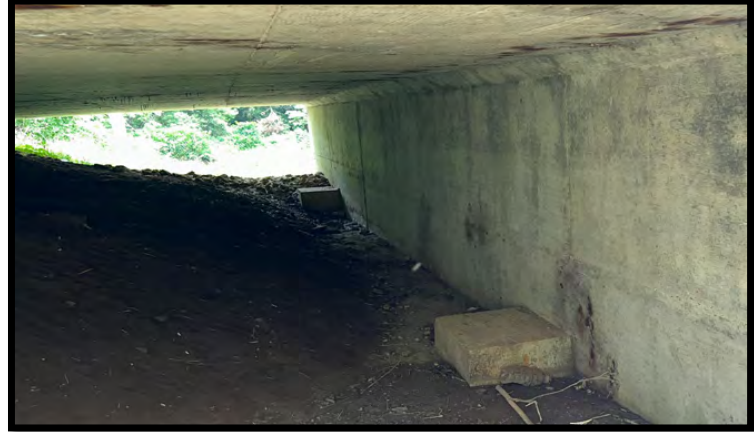
Photo 14: Looking southwest, under the bridge from the northeast corner of the bridge. There were no signs of bats or birds.
