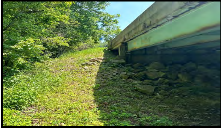
Photo 25: Looking southeast at the southwest corner of the bridge from the south bank of Big Blue River.
