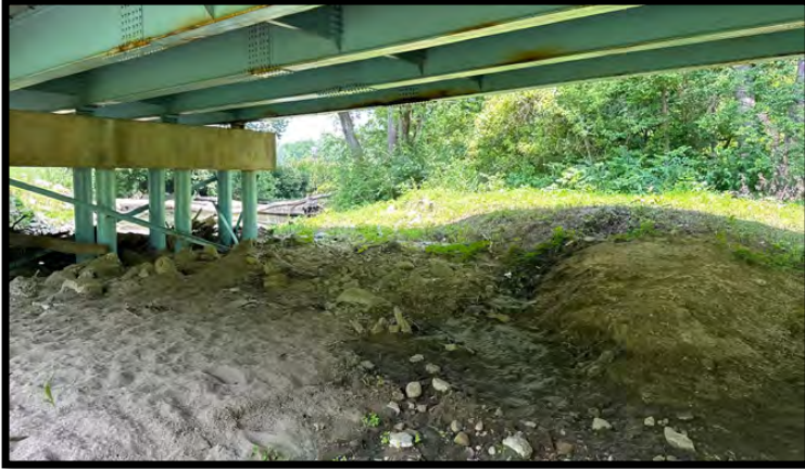
Photo 57: Looking southwest at the scour under the south end of the bridge.
