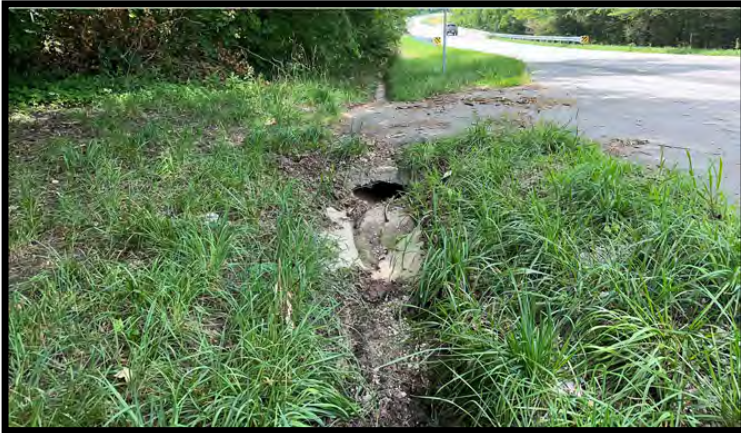
Photo 39: Looking northwest at the drive pipe along RSD3 that goes under the entrance to the road/path in the southwest investigated area.
