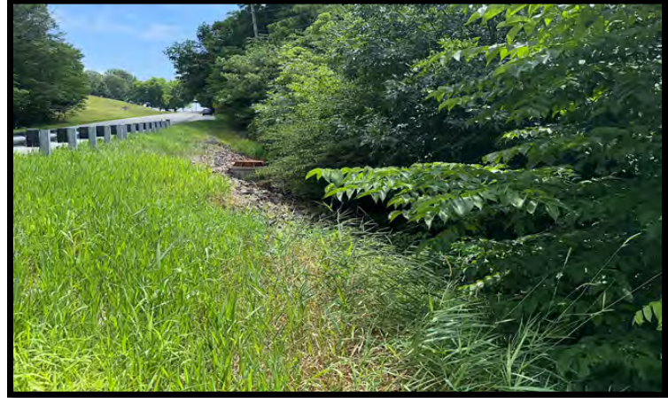
Photo 46: Looking southeast, upslope, along RSD3 as it comes along the southwest side of the bridge.
