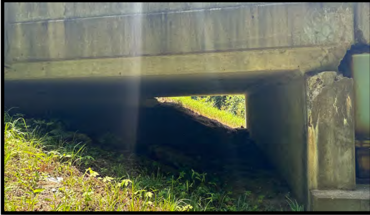
Photo 29: Looking southwest under the bridge from the southeast corner. There were no signs of birds or bats.
