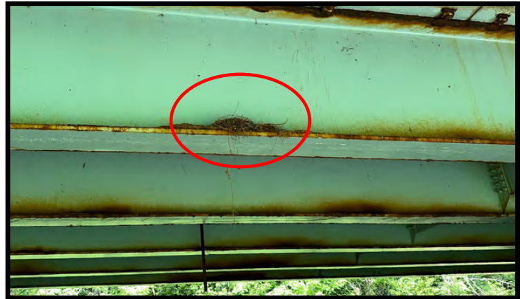
Photo 56: Looking southwest at the nest of an indeterminate species of bird under the south end of the bridge.
