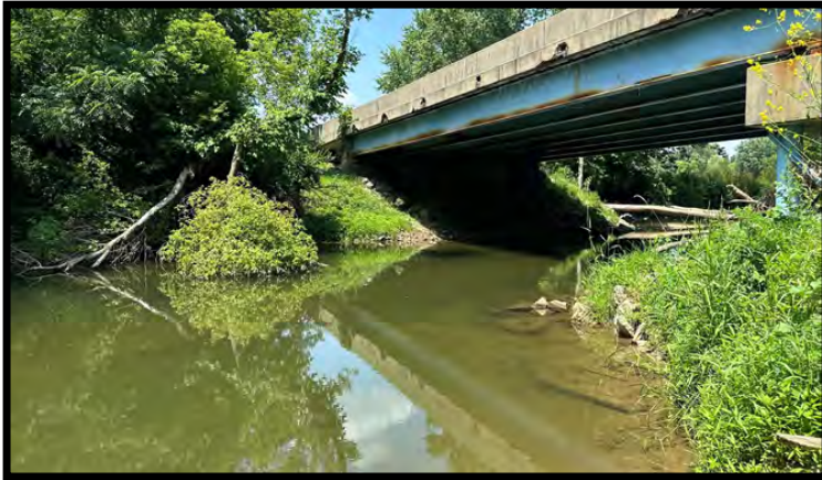
Photo 53: Looking north at the southwest (downstream) opening of the bridge from the south bank in southwest corner of the bridge.
