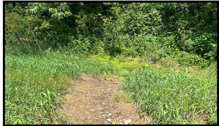
Photo 12: Looking northeast along the drainage from the northeast corner of the bridge.
