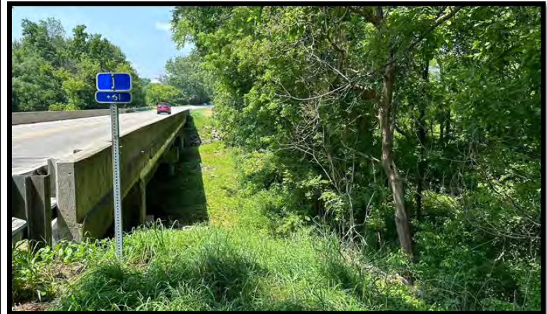
Photo 28: Looking northwest from the top of the southeast slope and southeast corner of the bridge.
