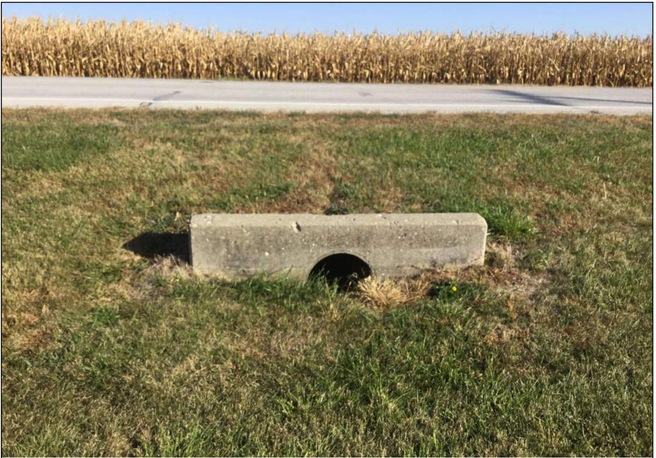
177. Looking north at Structure No. 110 located along the south side of SR 32. No stream or wetland features were observed. This structure will be replaced as part of this project. Photo taken October 8, 2020.
