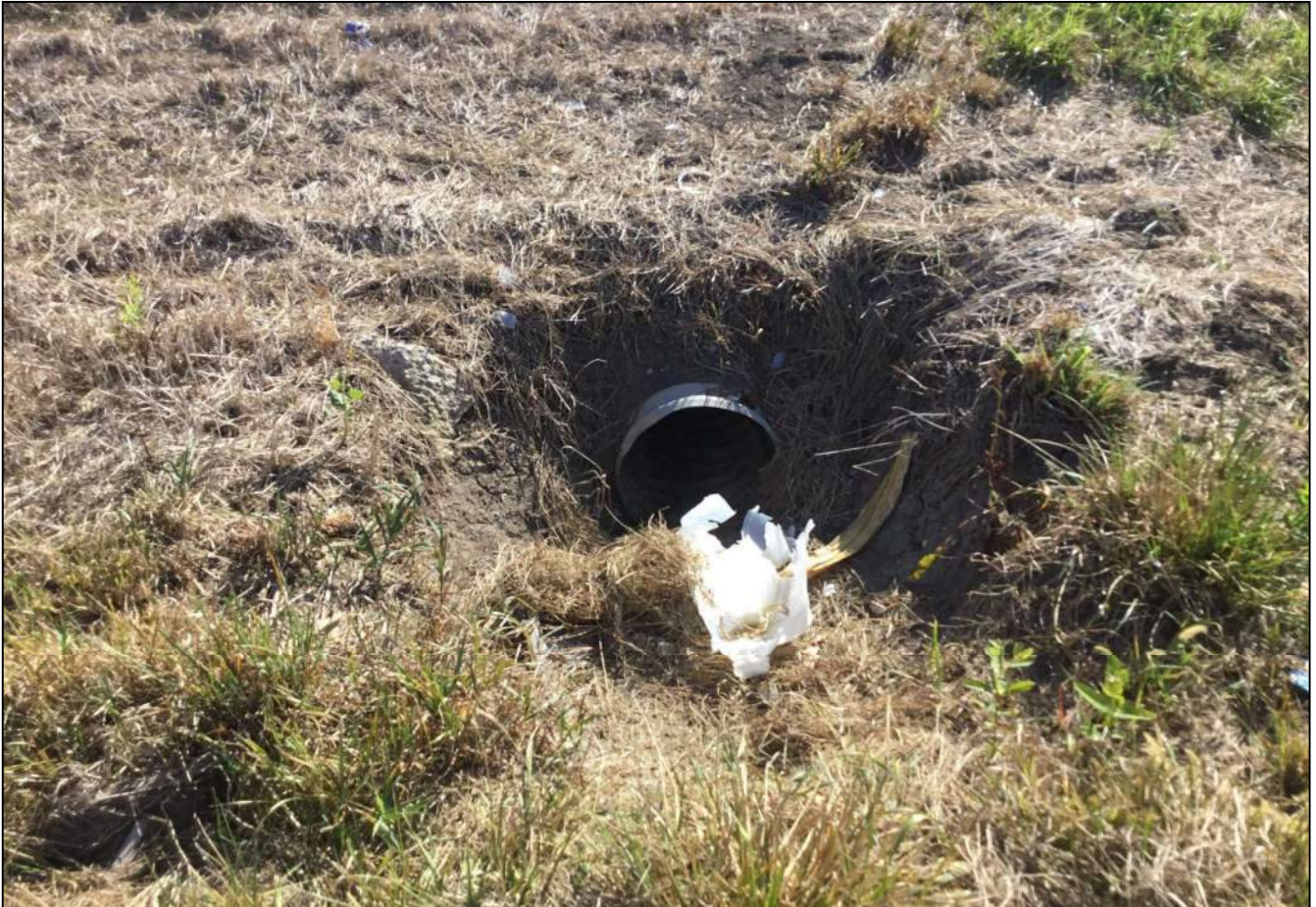
204. Looking south at Structure No. 102 located on the north side of SR 32. No stream or wetlands were found. Photo taken October 7, 2021.
