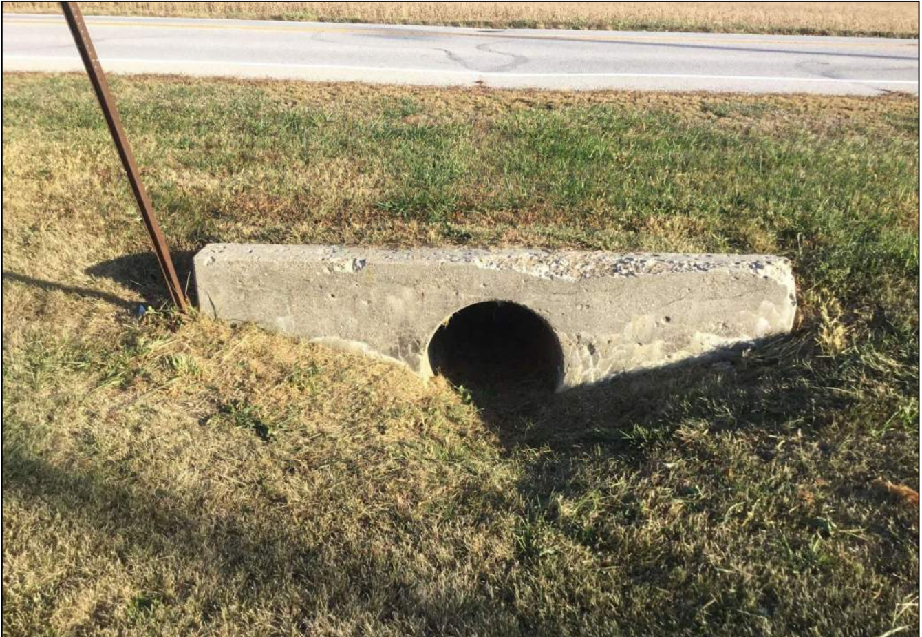
192. Looking north at Structure No. 103 along the south side of SR 32. No stream or wetland features were observed. This structure will be replaced as part of this project. Photo taken October 7, 2020.
