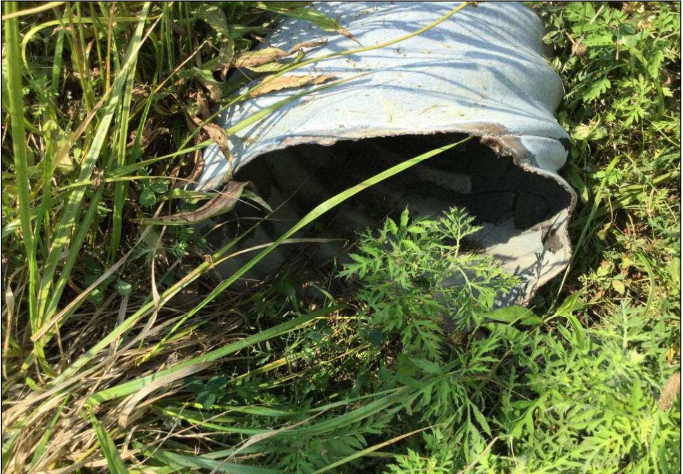
202. Looking north at Structure No. 102 located on the south side of SR 32. No stream or wetlands were found. This structure will be replaced as part of this project. Photo taken July 6, 2021.
