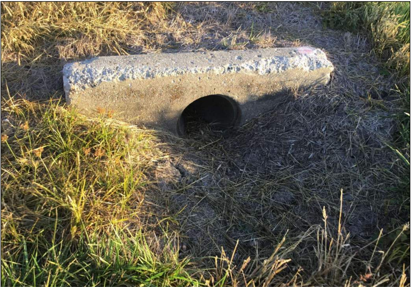
207. Looking northeast at Structure No. 101 located on the south side of SR 32. No stream or wetlands were observed. This structure will be replaced as part of this project. Photo taken October 8, 2020.
