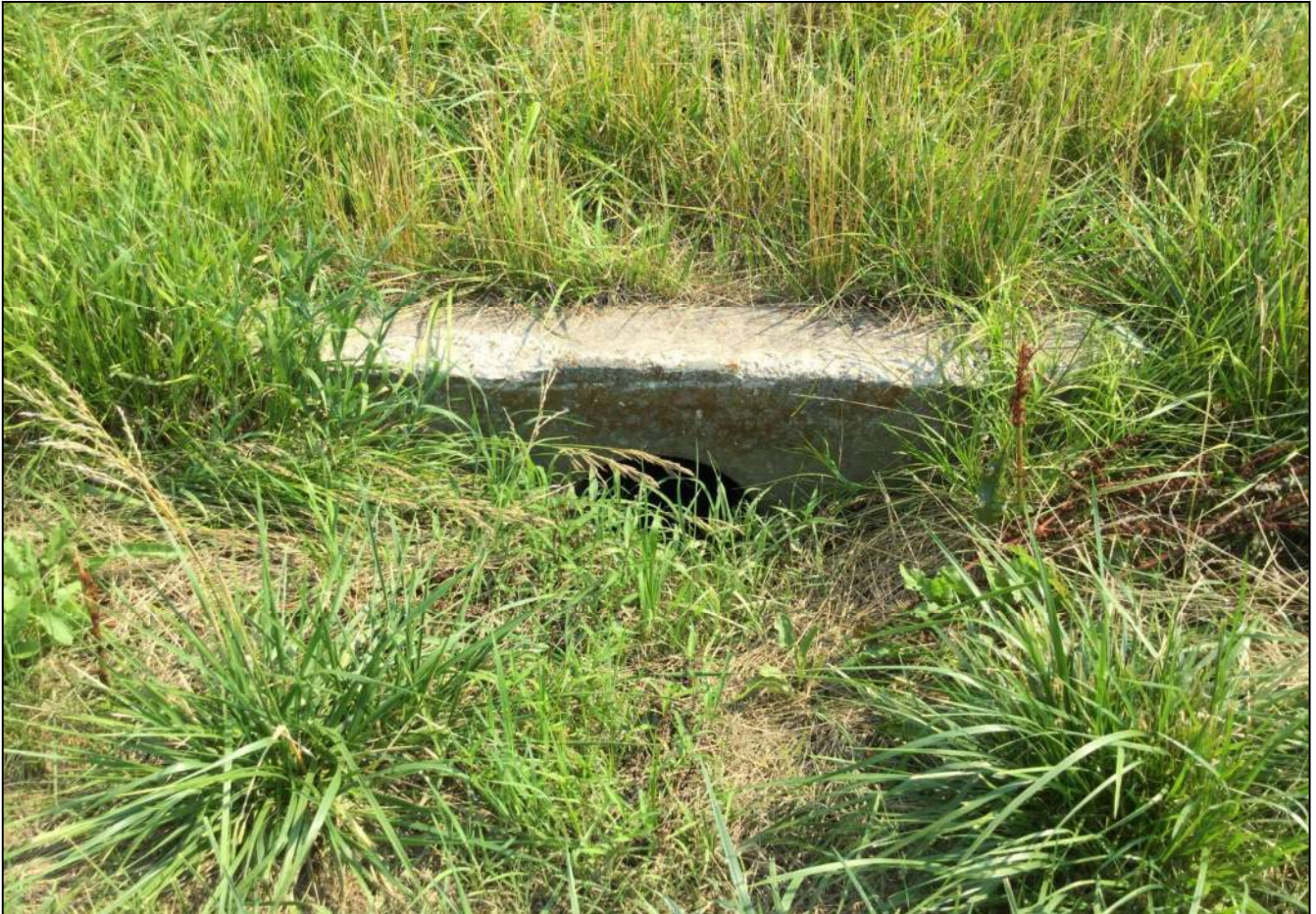
208. Looking south at Structure No. 101 located on the north side of SR 32. No stream or wetlands were found. Photo taken July 6, 2021.
