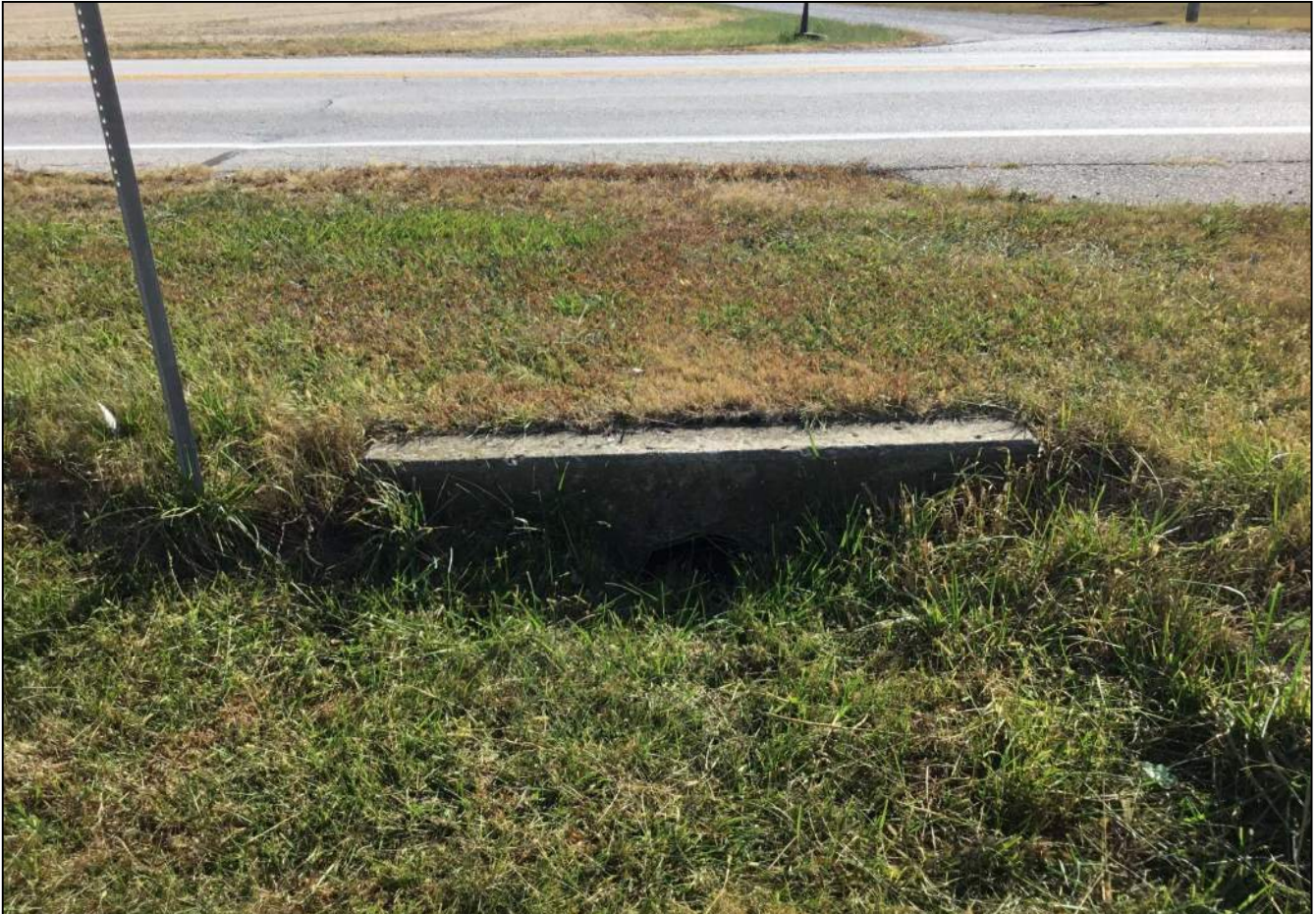
186. Looking southwest at Structure No. 104 that is partially buried. No stream or wetland features were observed. This structure will be replaced as part of this project. Photo taken October 7, 2020.
