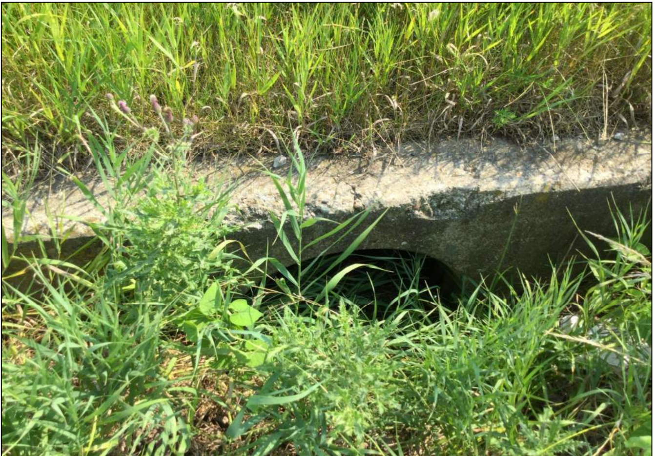
193. Looking south at Structure No. 103 located on the north side of SR 32. No stream or wetlands were observed. Photo taken July 6, 2021.
