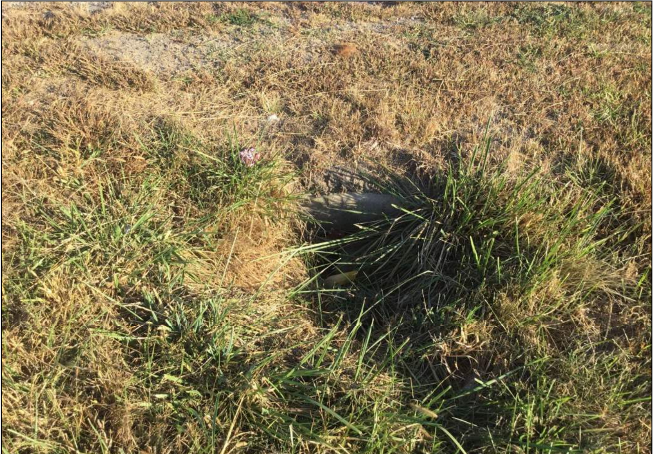
188. Looking north at Structure No. 104 located on the south side of SR 32 that conveys drainage underneath SR 32 just east of CR 1075 W. Photo taken October 7, 2020.
