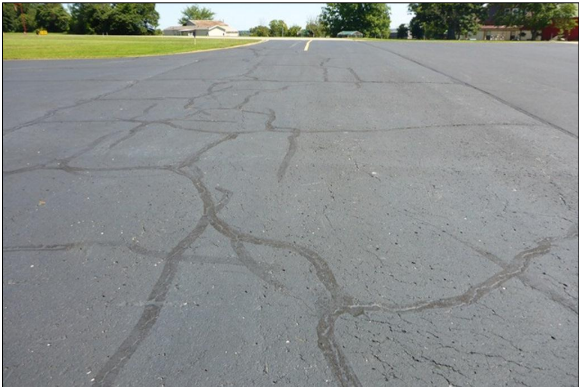
Figure 2-5. Typical AC Pavement in Poor Condition (Feature 4120)
