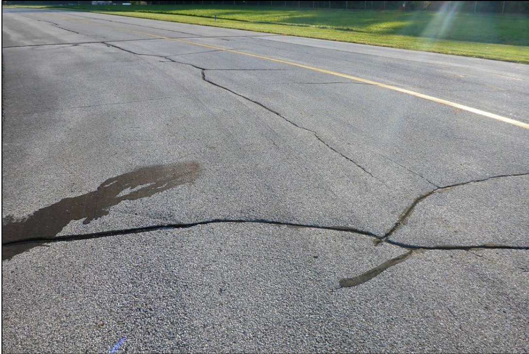
Figure 2-6. Typical AC Pavement in Poor Condition (Feature 130)
