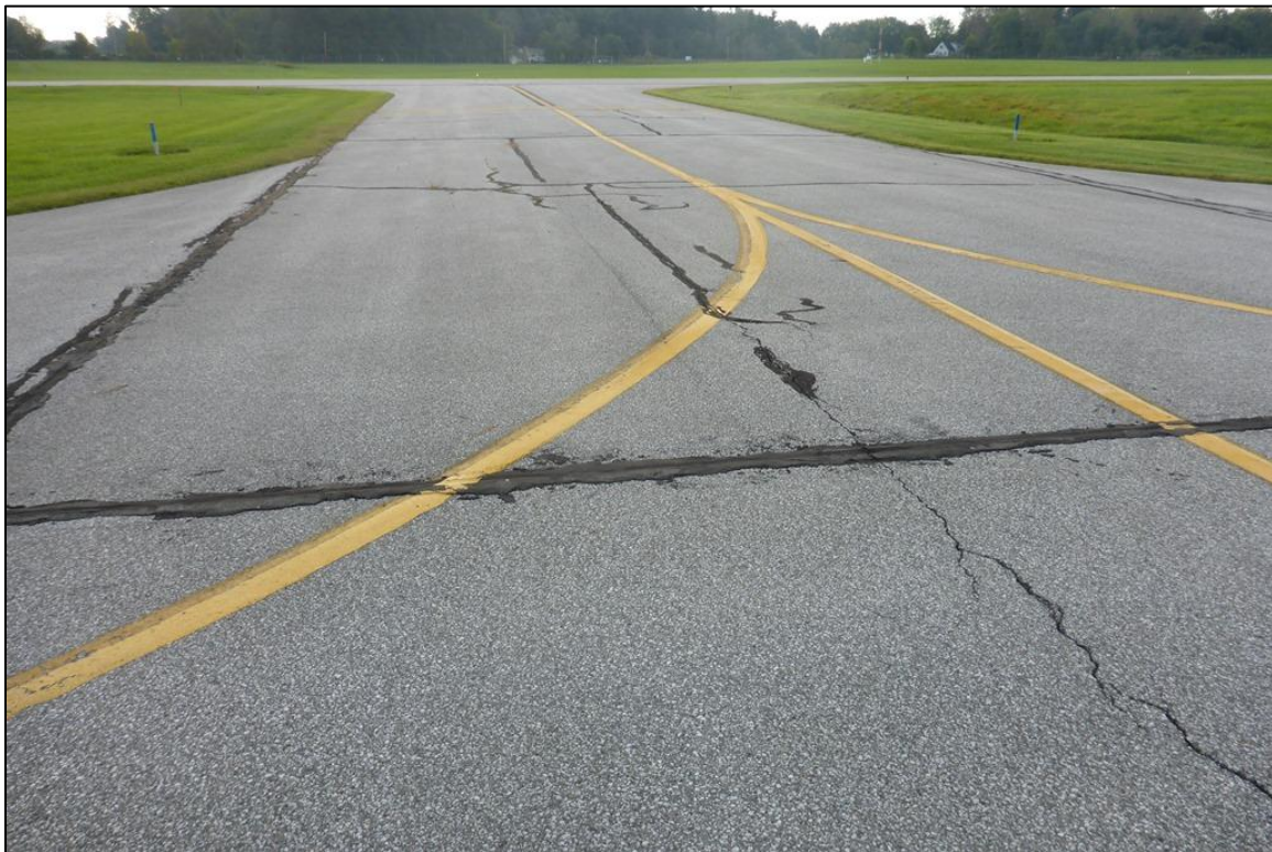
Figure 2-5. Typical AC Pavement in Fair Condition (Feature 325)
