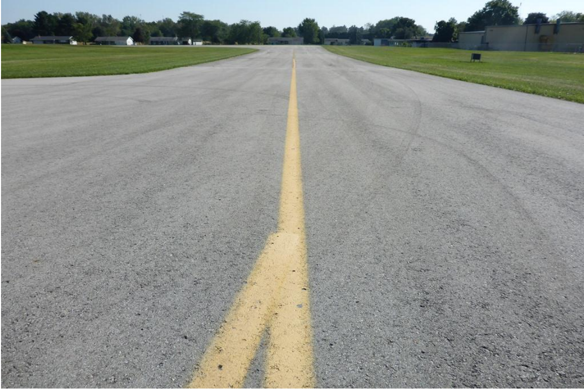
Figure 2-4. Typical AC Pavement in Poor Condition (Feature 110)
