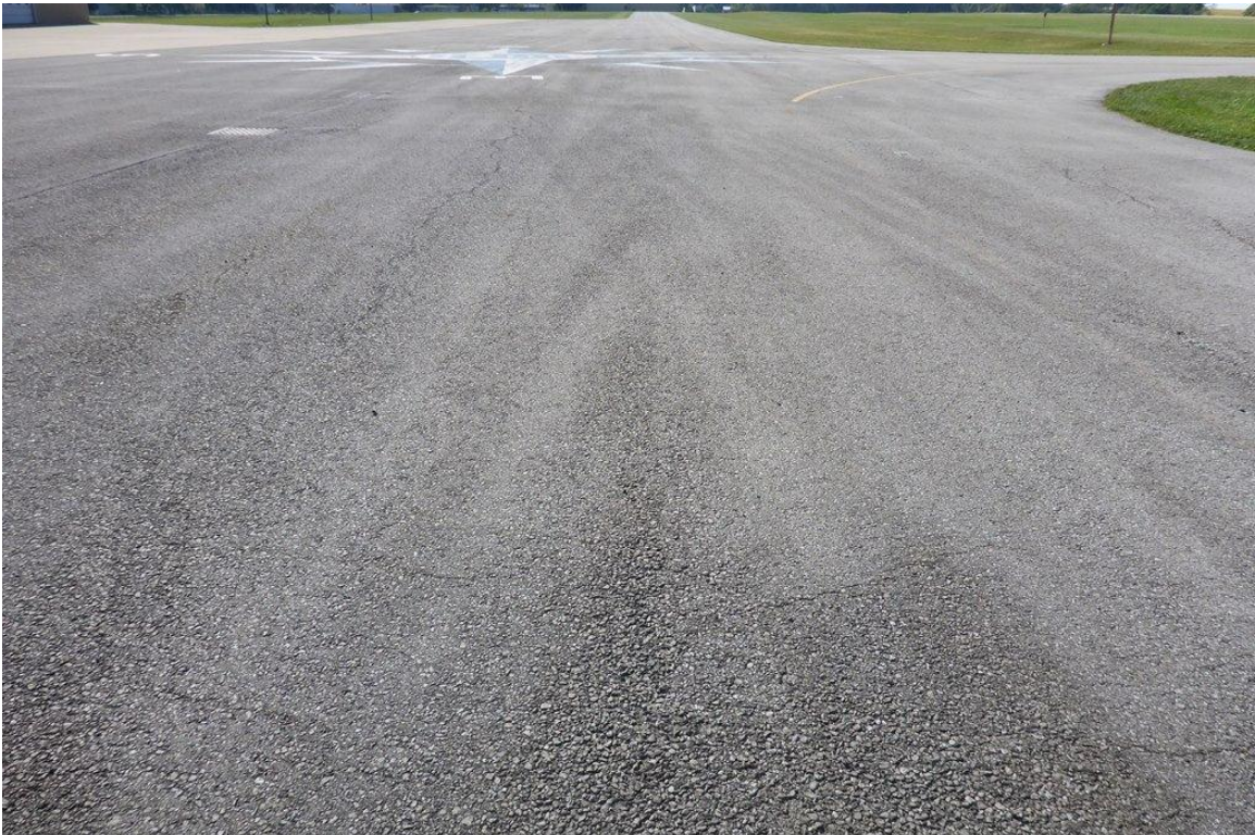
Figure 2-5. Typical AC Pavement in Poor Condition (Feature 3005)
