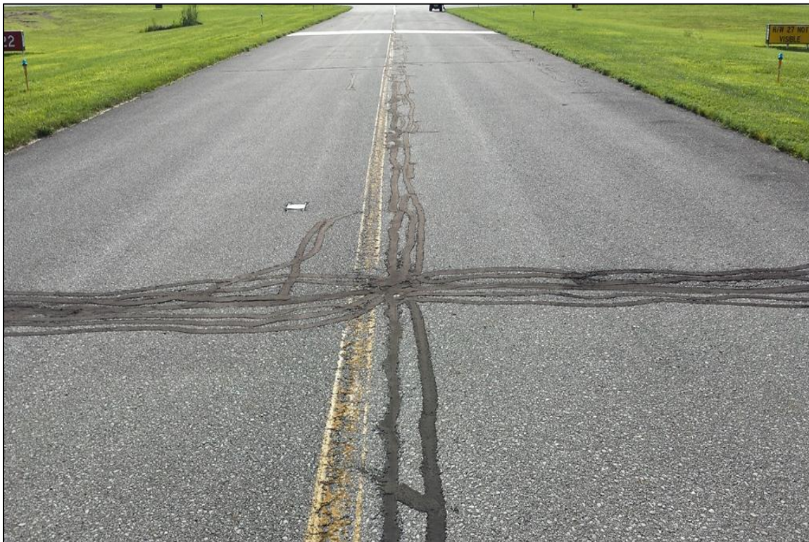
Figure 2-5. Typical AC Pavement in Fair Condition (Feature 101)
