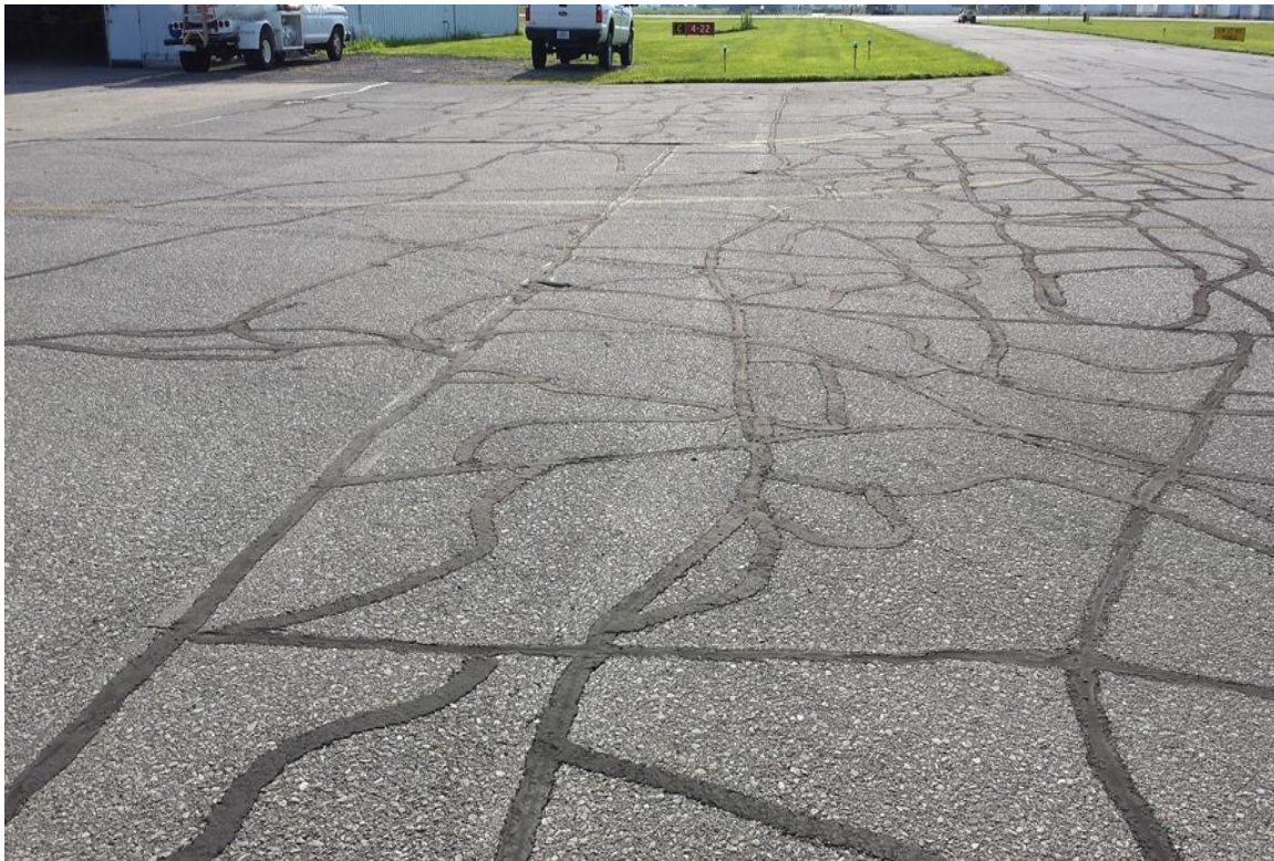
Figure 2-6. Typical AC Pavement in Poor Condition (Feature 210)
