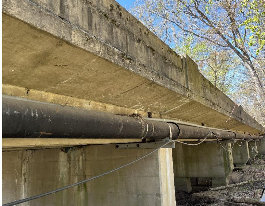
Photo: 1 Vantage Point: Under structure just north of Span E Direction: Looking southwest Description: North elevation
