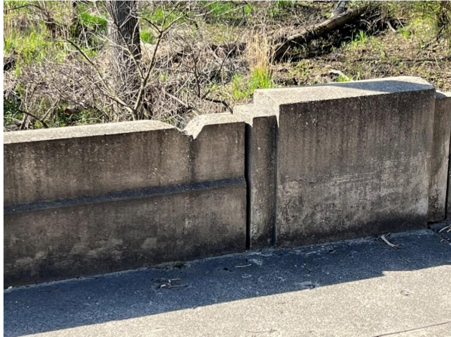
Photo: 7 Vantage Point: Bridge deck Direction: Looking south Description: Chipped section of south bridge railing
