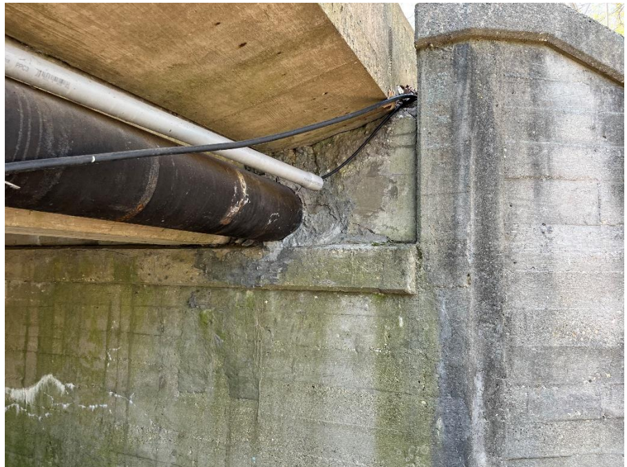
Photo: 14 Vantage Point: Just north of Span A under bridge Direction: Looking west Description: Utilities through Abutment 1
