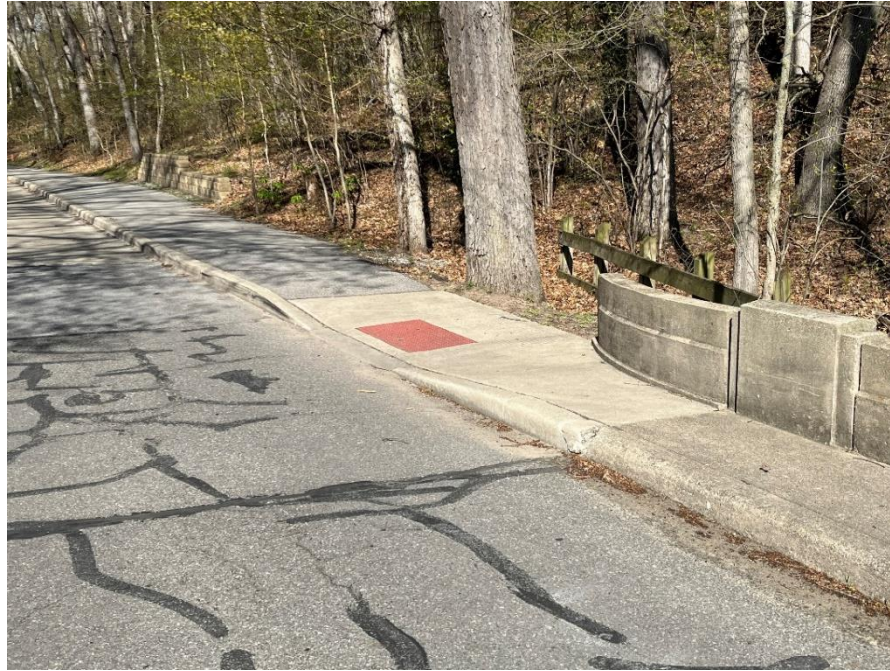
Photo: 11 Vantage Point: Bridge deck Direction: Looking west Description: Northwest curb ramp and bridge railing transition
