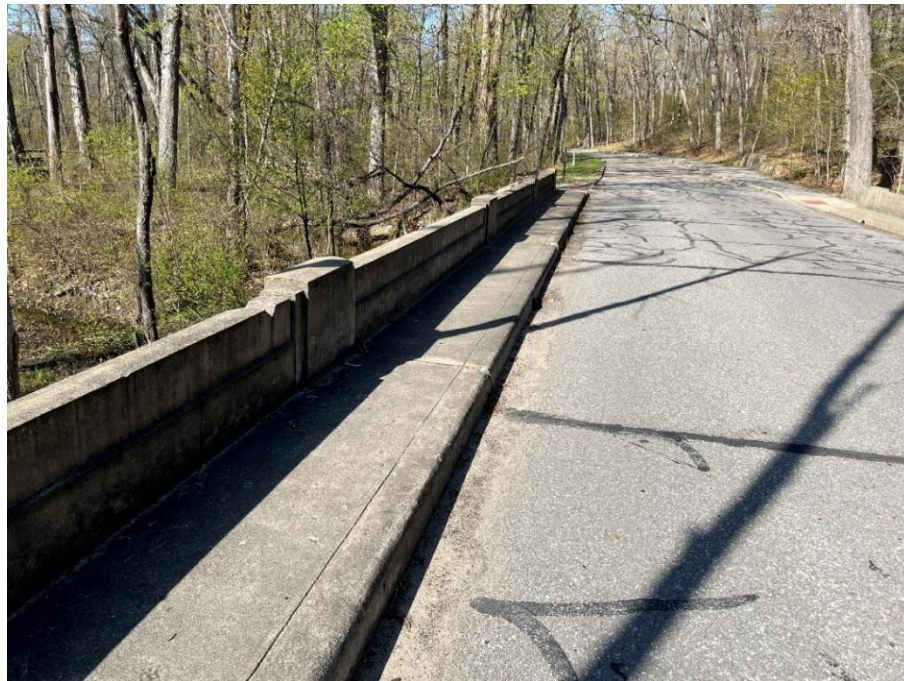
Photo: 6 Vantage Point: Bridge deck Direction: Looking west Description: South bridge railing and sidewalk
