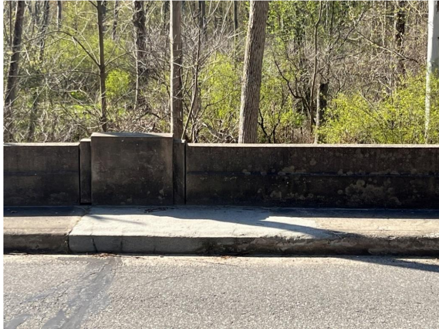
Photo: 5 Vantage Point: bridge deck Direction: Looking south Description: South sidewalk patching
