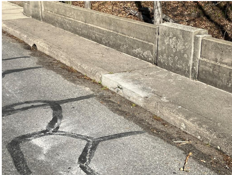
Photo: 8 Vantage Point: Bridge deck Direction: Looking northwest Description: North sidewalk patch
