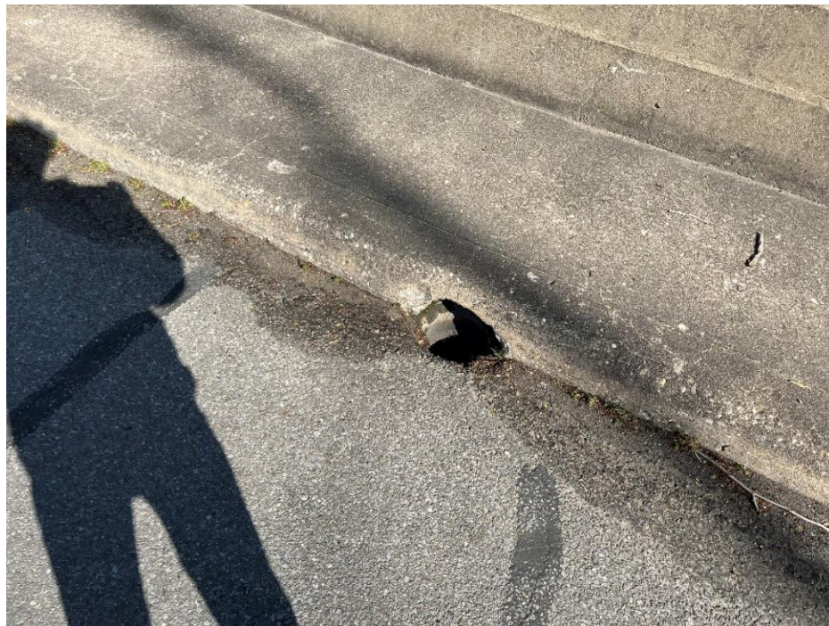
Photo: 4 Vantage Point: North side of bridge deck Direction: Looking north Description: Typical deck drain
