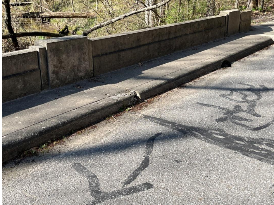
Photo: 9 Vantage Point: Bridge deck Direction: Looking southwest Description: South sidewalk chipping
