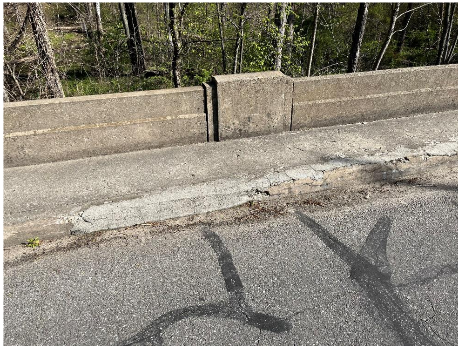
Photo: 10 Vantage Point: Bridge deck Direction: Looking north Description: North sidewalk spalling
