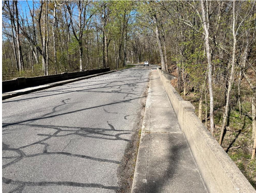
Photo: 3 Vantage Point: East side of bridge Direction: Looking west Description: Bridge deck, north Sidewalk, north bridge rail
