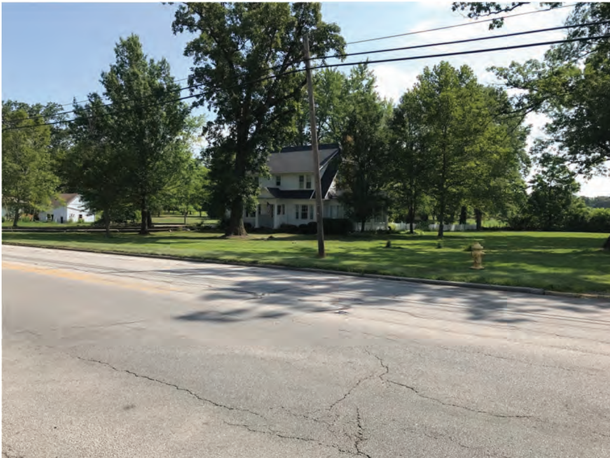
20. Looking NE at the intersection of US 27 (Meridian Street) and Meridian Heights
