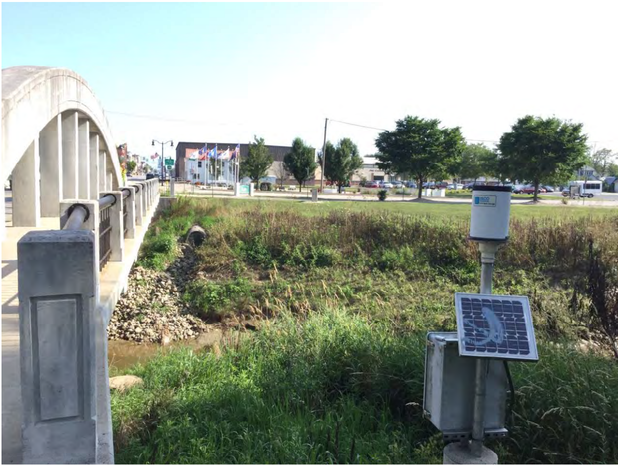
7. Looking north from the top of the upstream right bank towards culvert outlet.
