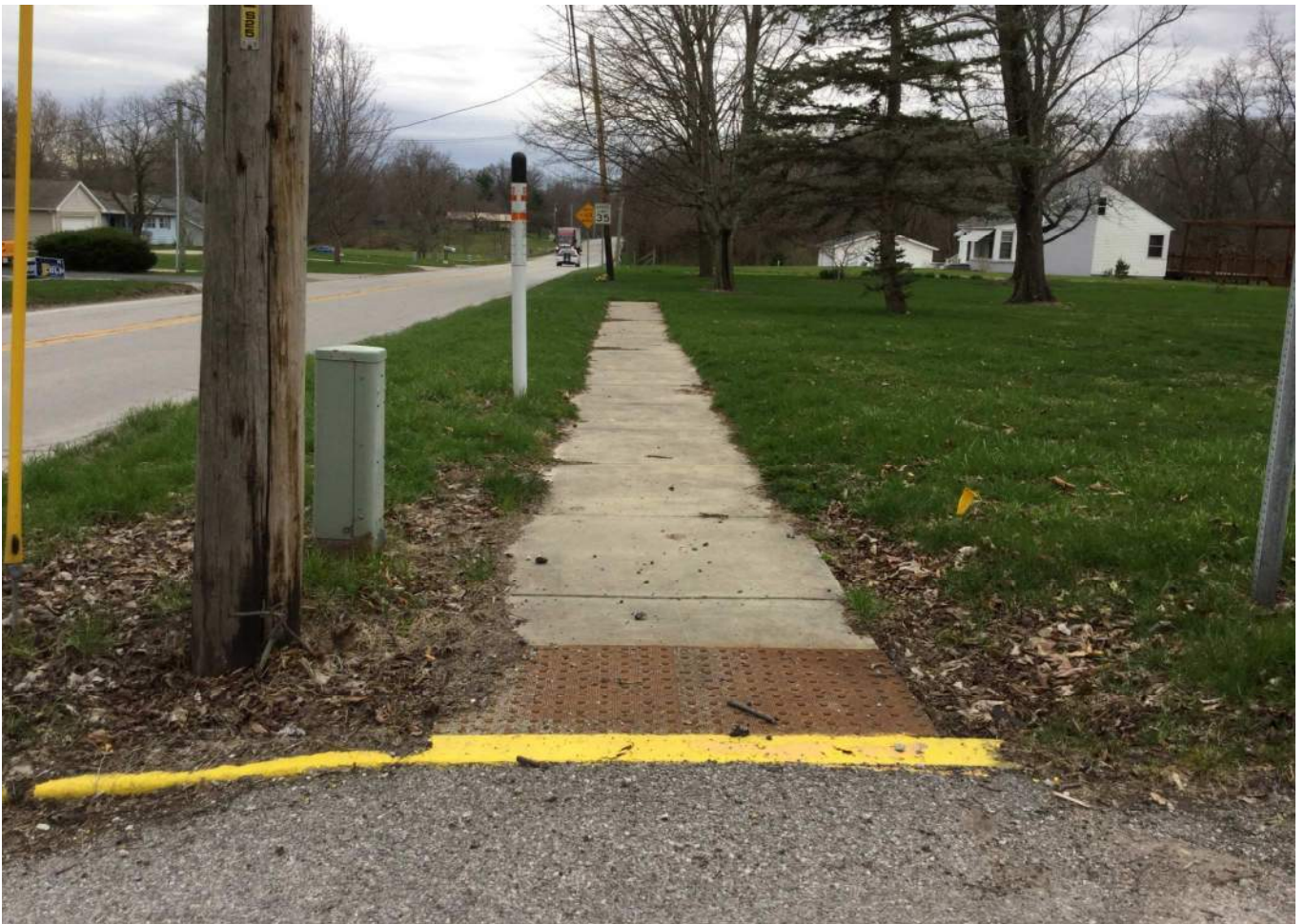
38. Looking south from the SR 43 / West 10 th Street Intersection at termination of existing sidewalk and curb ramp along the west side of SR 43.
