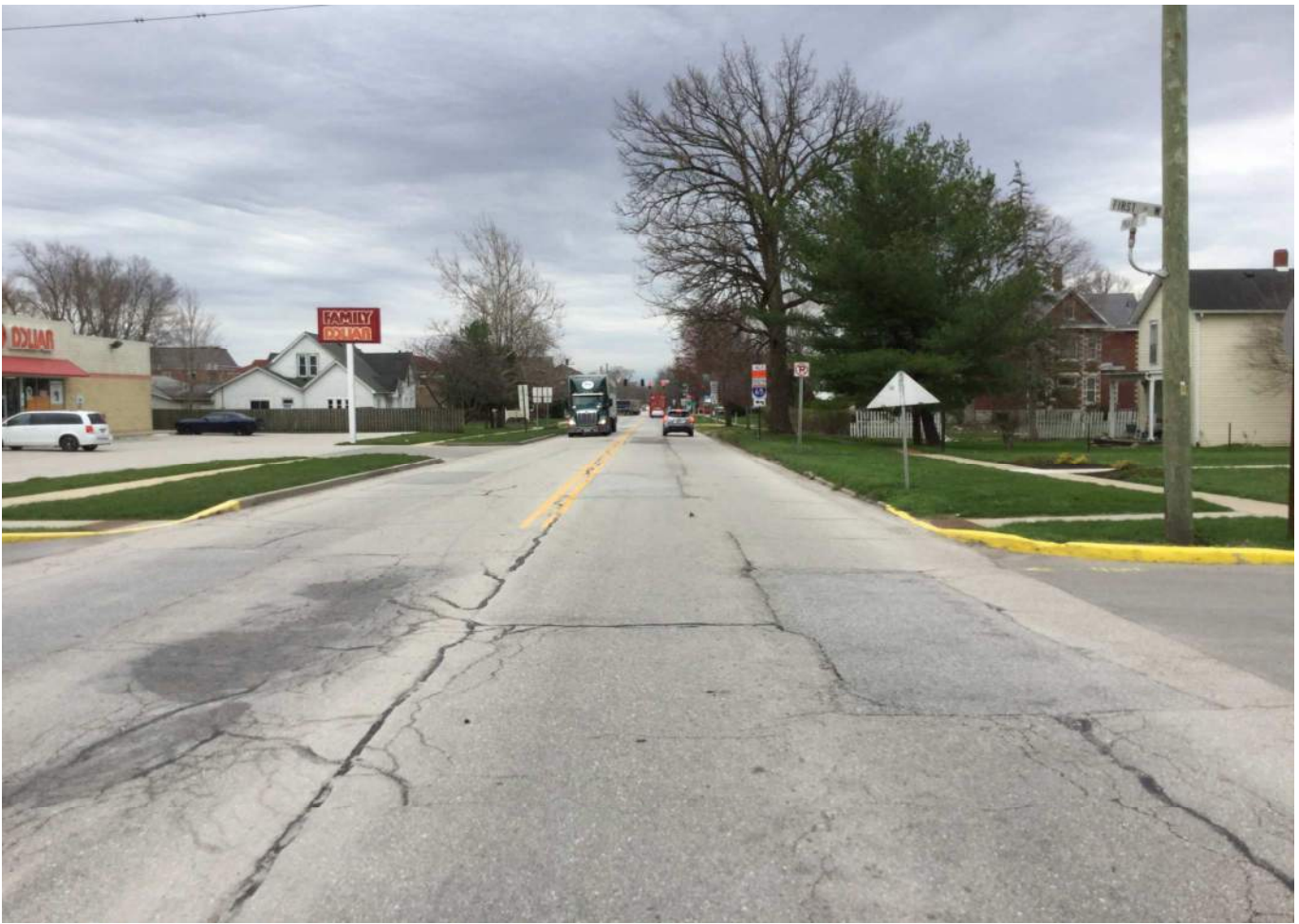
13. Looking south from the SR 18 / West 1 st Street Intersection at roadway and adjacent landscape.
