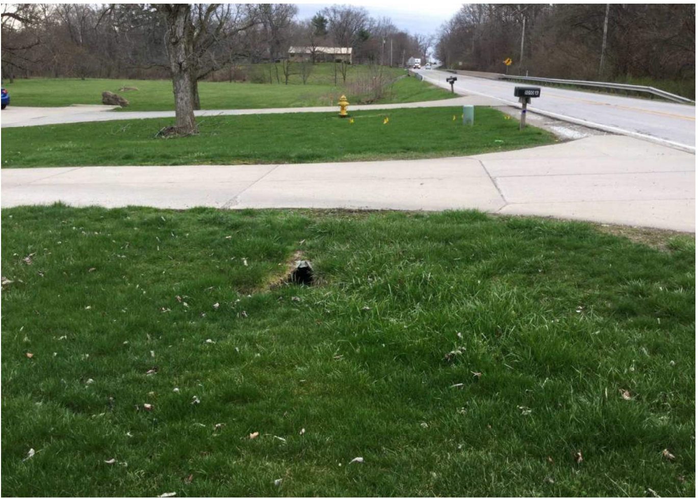
41. Looking south along the east side of SR 43 at a small driveway pipe and adjacent landscape.
