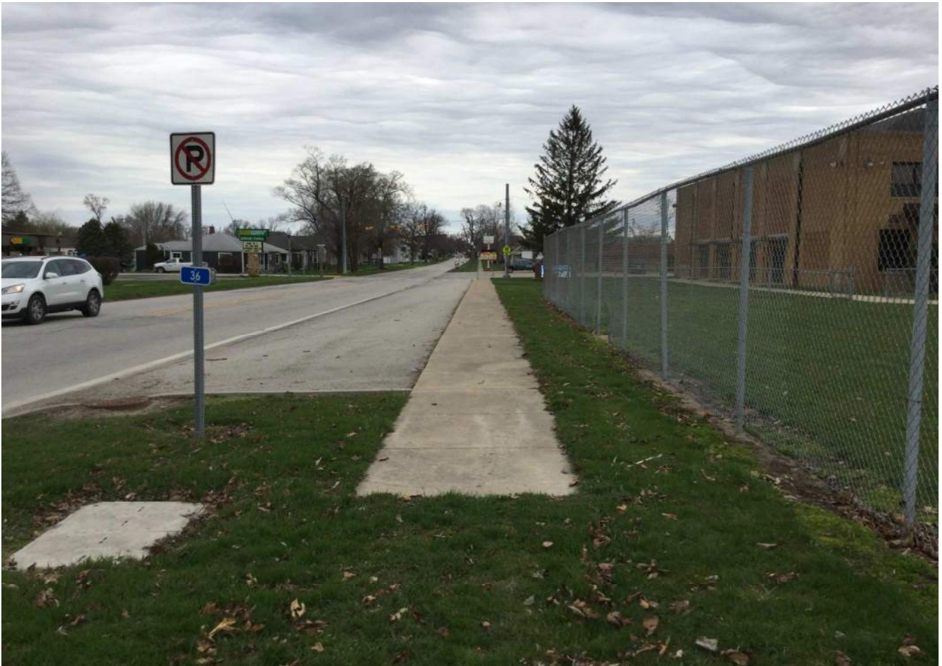
34. Looking northwest from Frontier Elementary School at sidewalk terminating along the east side of SR 43.
