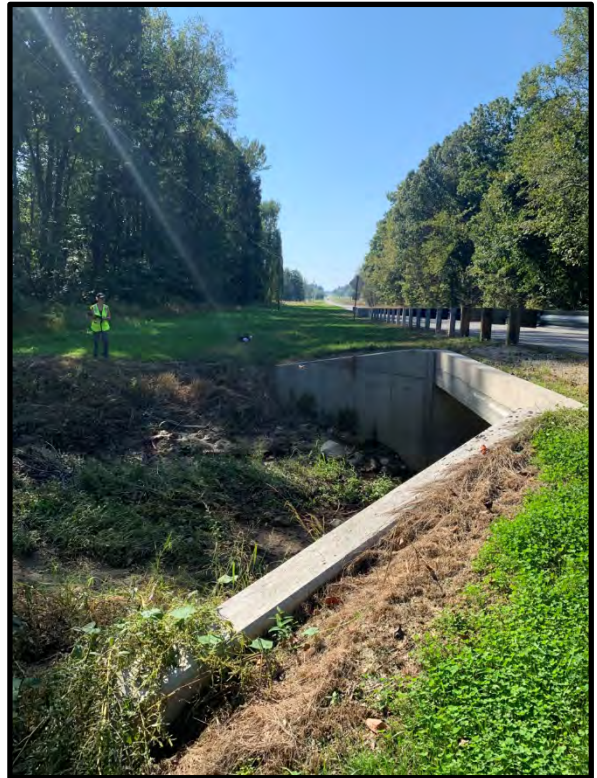
4. View of new box culvert at unnamed tributary to White Creek on the south side of SR 258, looking west. 9/28/2021
