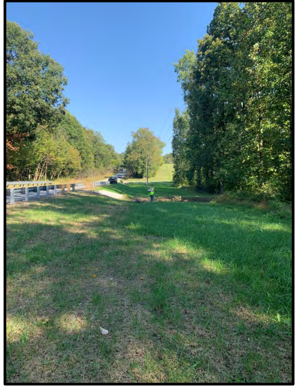
3. View of mowed ROW and new box culvert along the south side of SR 258, looking east. 9/28/2021
