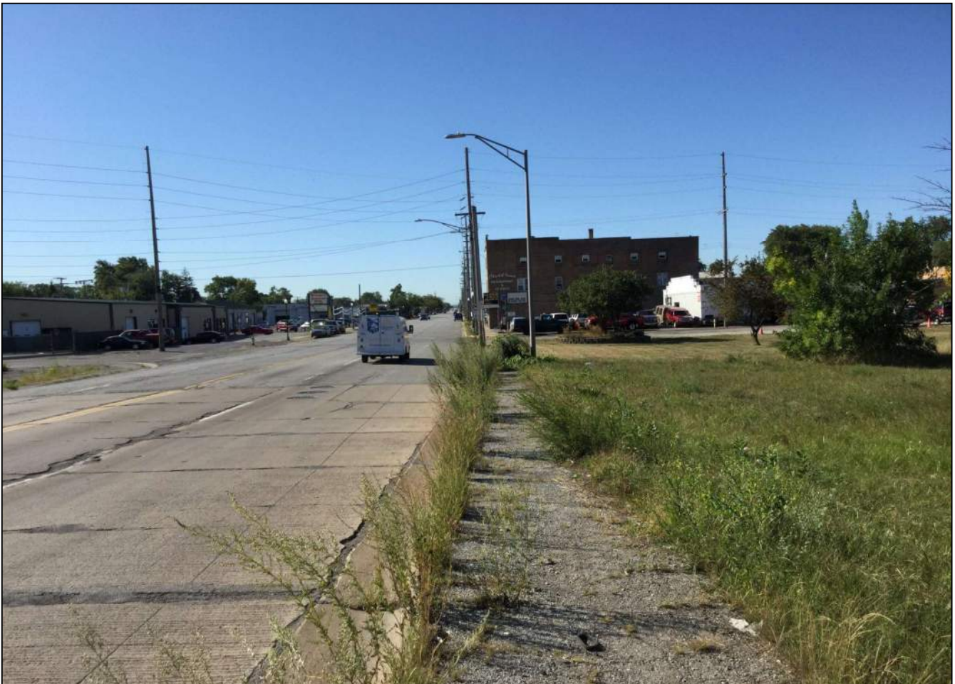
35. Looking south along the west side of Kennedy Ave. at the V gutter present and gravel shoulder.
