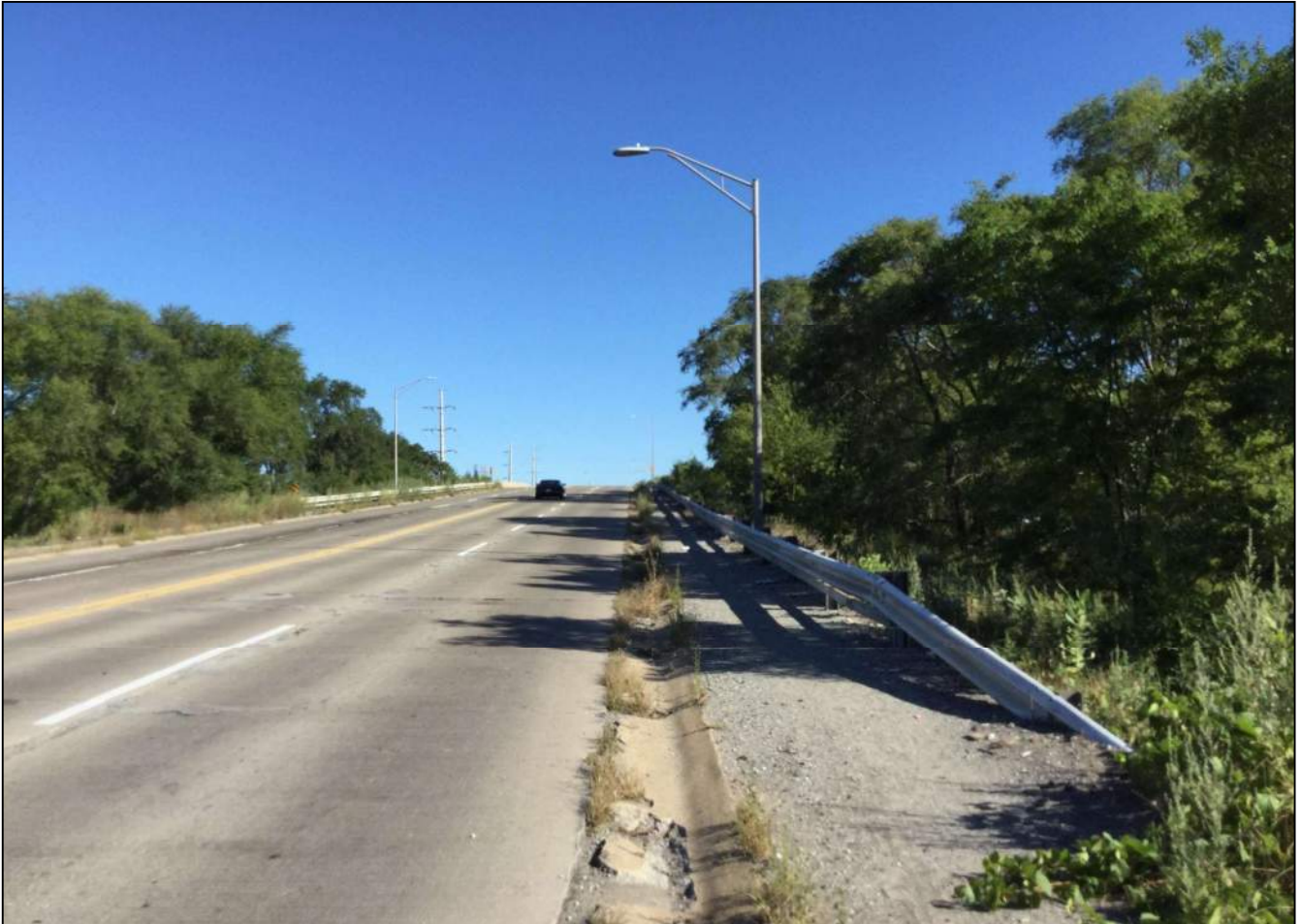
34. Looking north along the east side of Kennedy Ave. at the V gutter present and gravel shoulder.
