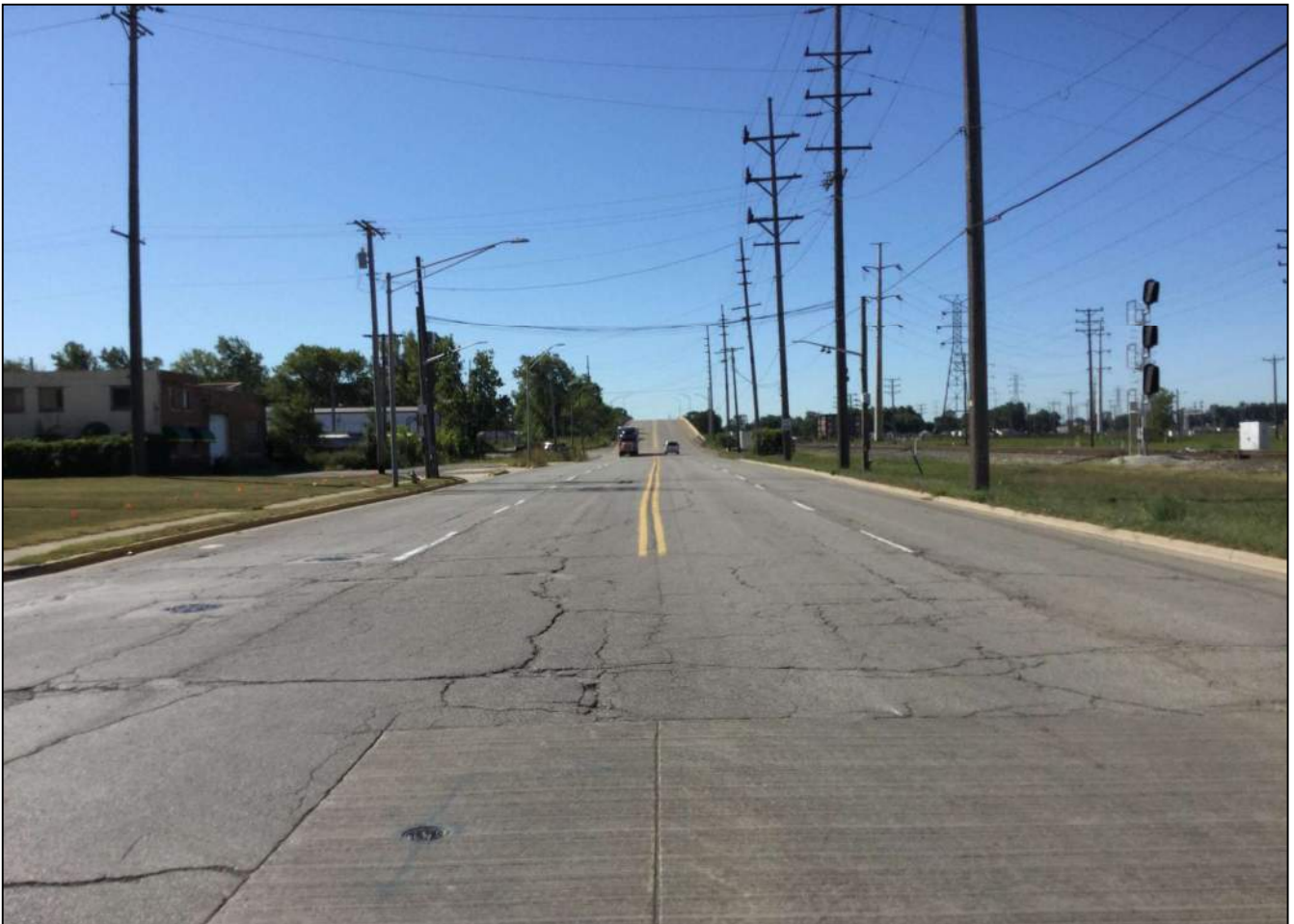
47. Looking south down the center of Kennedy Ave. just west of the south access road for US20/Michigan St.
