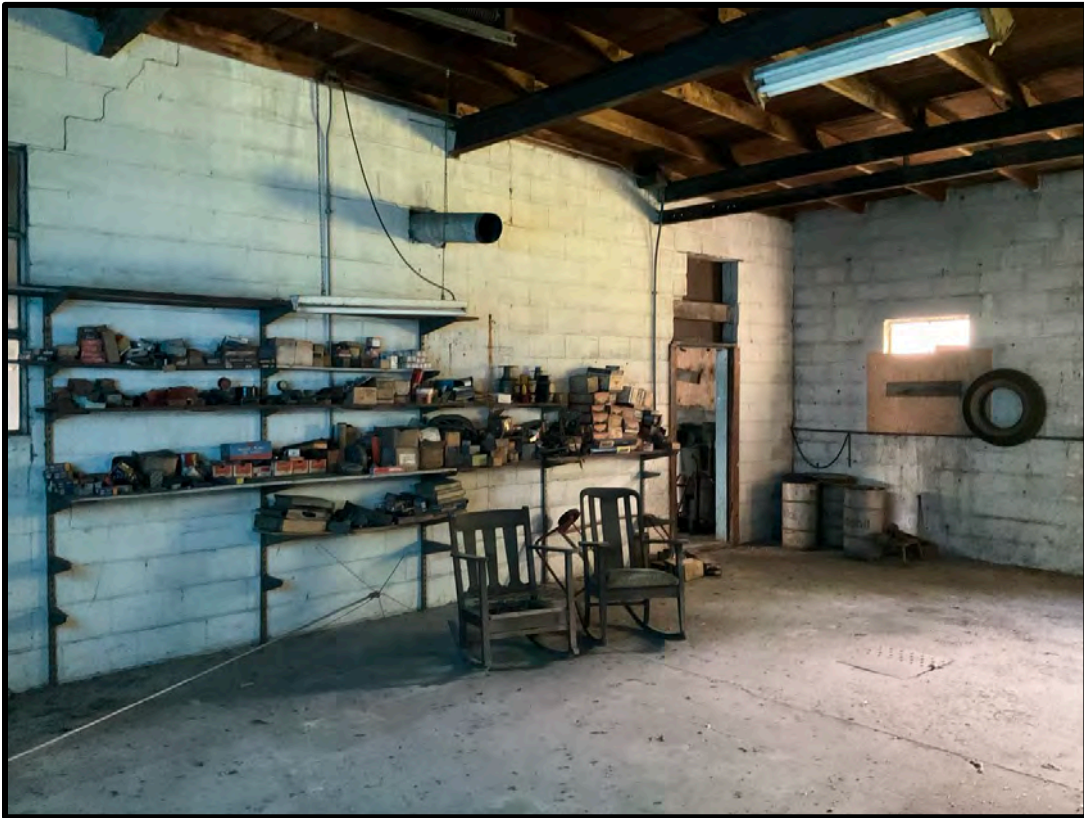
Figure 5: Looking SE inside Lochmueller #1 in W service bay
