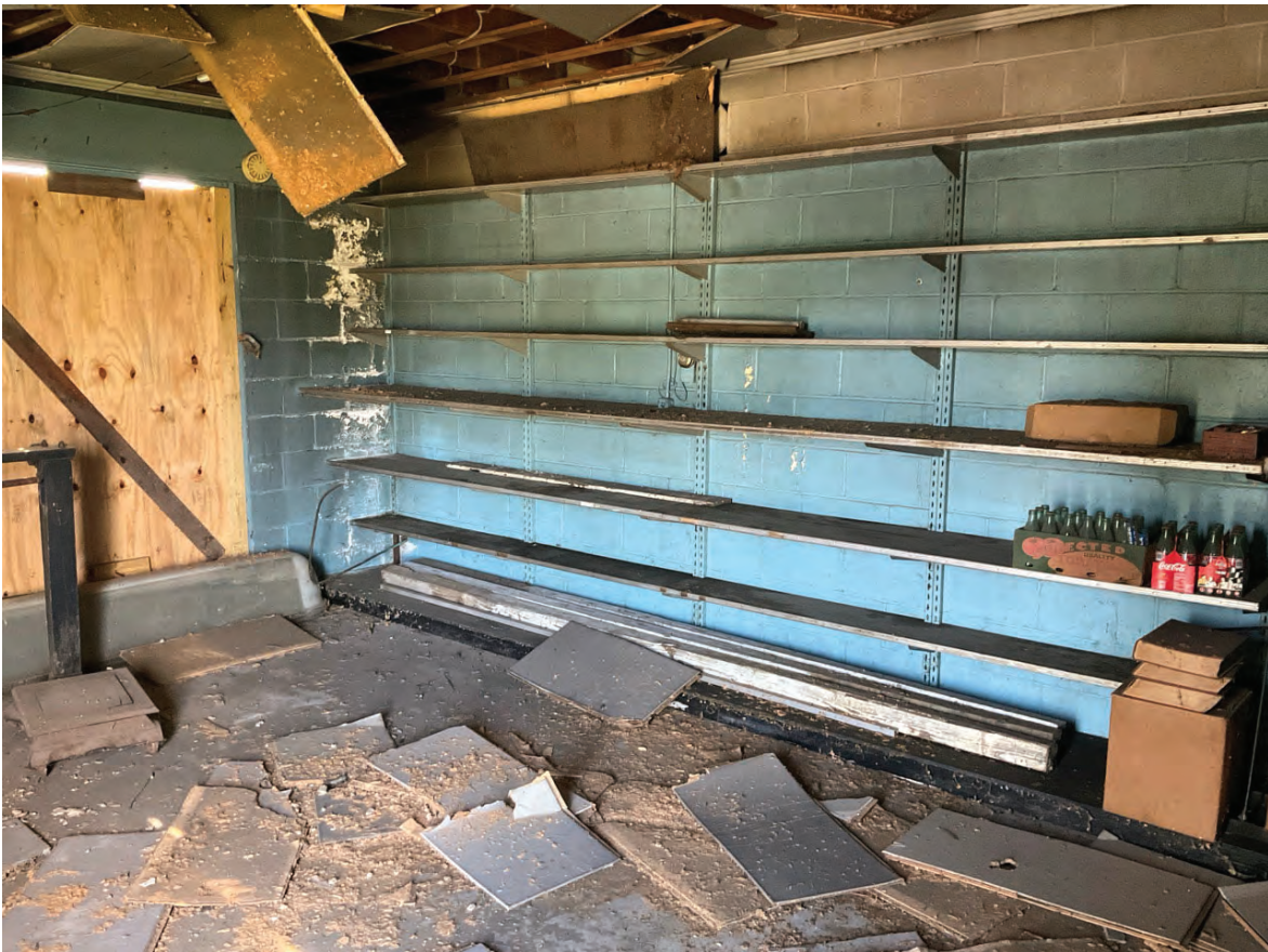
12. Looking SE in service counter area E bay in Lochmueller #1 (Contributing, 2904 S 1050 E)
