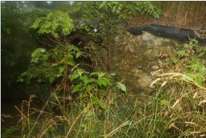
Photograph 3. View of structure outlet. Photo taken on the southside of SR 58, facing southwest.
