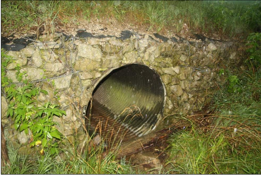
Photograph 1. View of structure inlet. Photo taken on the northside of SR 58, facing southeast.
