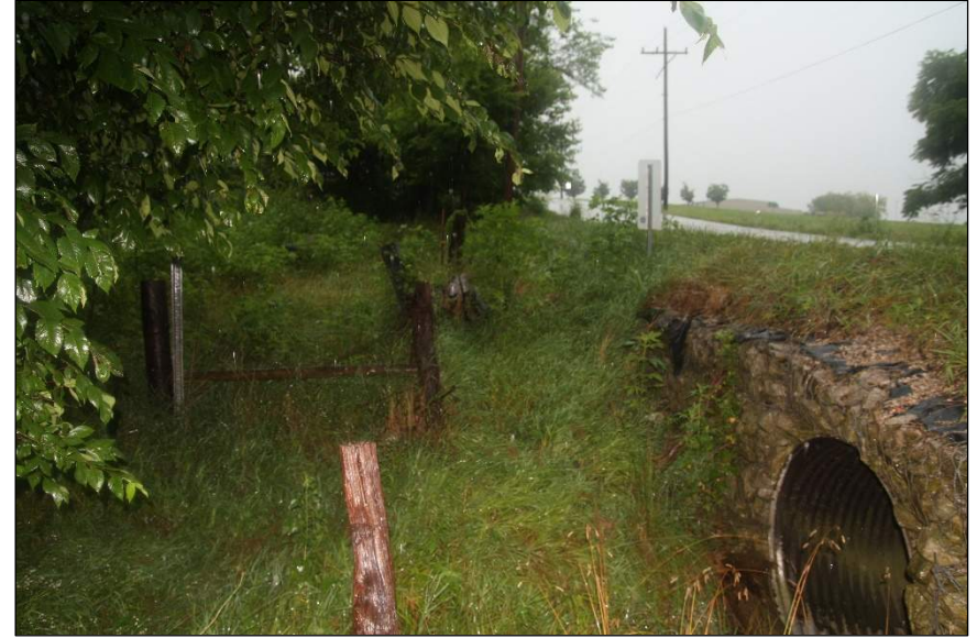
Photograph 2. View of structure inlet and vegetation within right-of-way. Photo taken on northside of SR 58, facing southeast.
