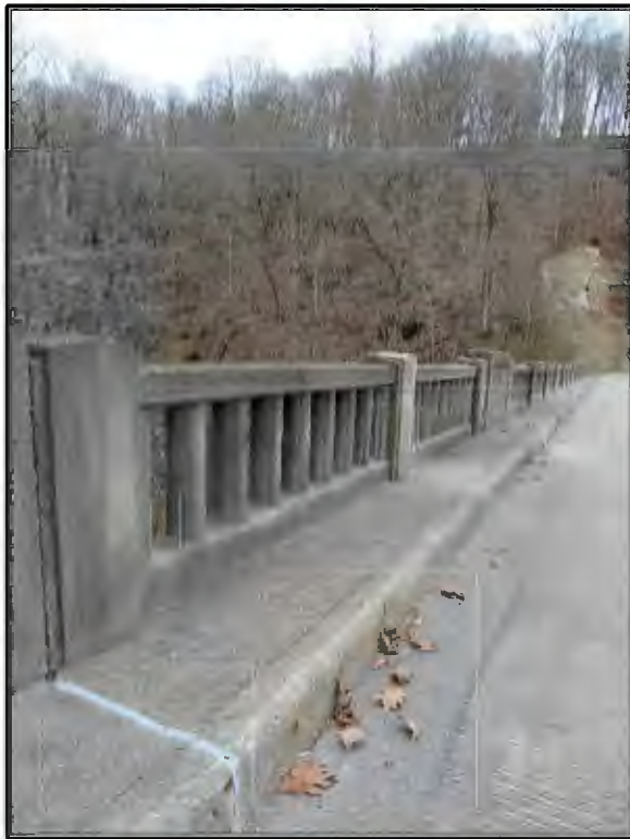
Figure 9. Concrete railing along the north side of the bridge (P000-39-06876B; NBI No. 60290), looking northeast.
