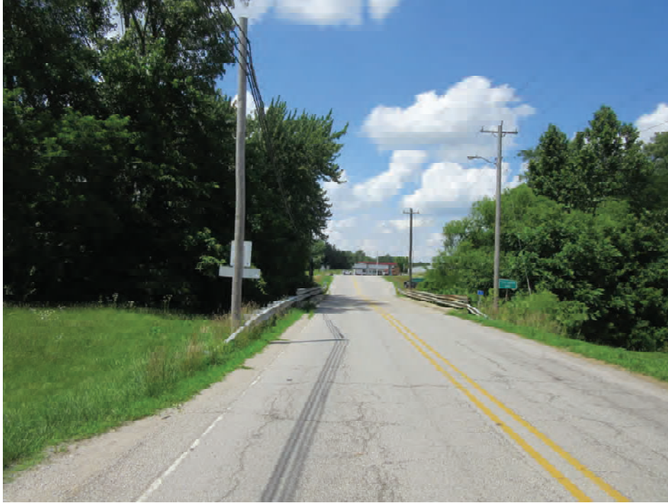
17. From just south of Structure No. 059-54-05061 looking north at SR 59 (Cross Street) and structure number 059-54-05061
