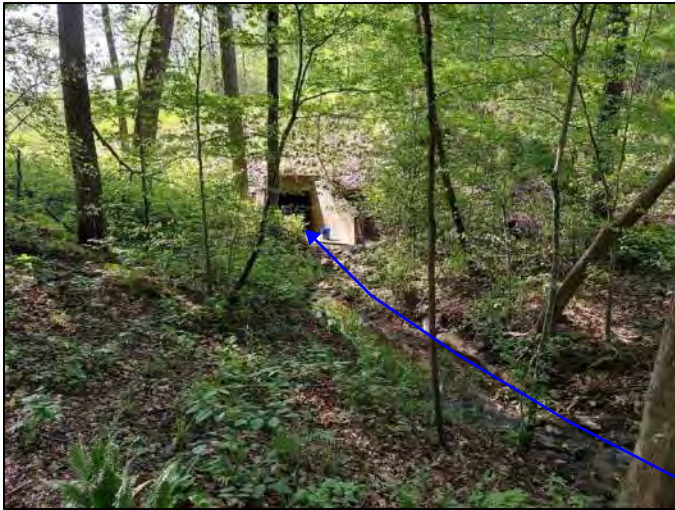
Photo 41. Outlet of culvert (CV 445-28-000.52) and UNT 1 to Beech Creek, facing downstream, viewing southeast, 5/13/2022
