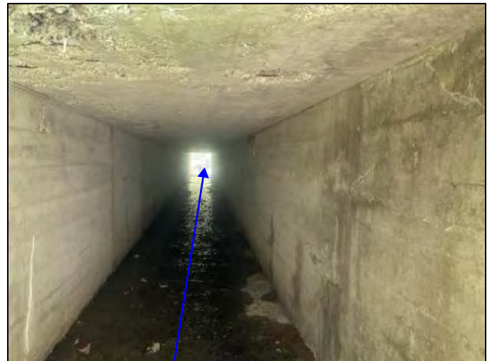
Photo 44. Looking through culvert (CV 445-28-000.52) at inlet with UNT 1 to Beech Creek, facing downstream, viewing southeast, 5/13/2022
