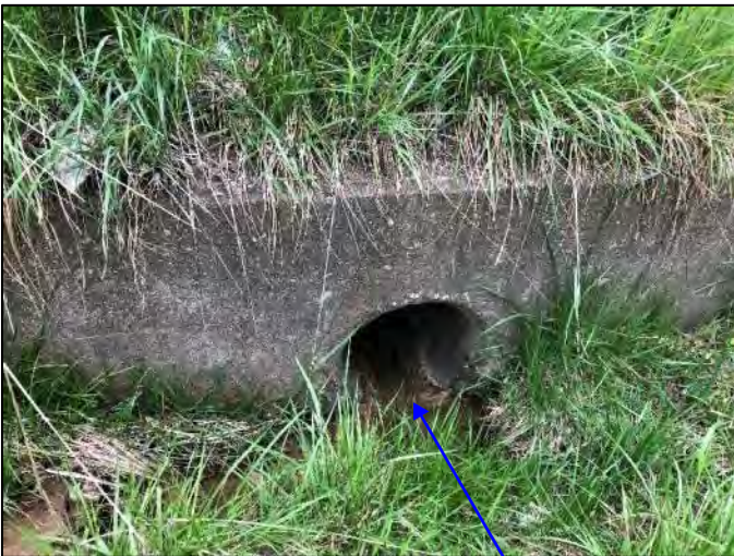
Photo 19. Looking through CLV-67652 at inlet with UNT 2 to Beech Creek, facing downstream, viewing north, 5/13/2022
