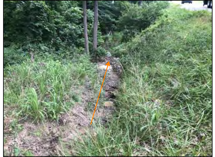
Photo 2. RSD 1 and eroded soils north of SR 445, viewing east, 7/7/2022
