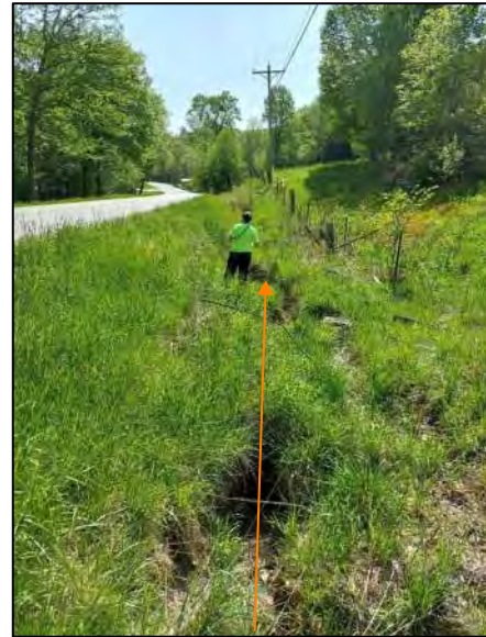
Photo 18. RSD 4 with heavy erosion, viewing east, 5/13/2022
