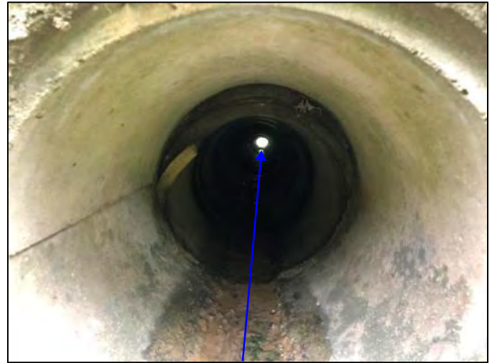
Photo 20. Inlet of CLV-67652 with UNT 2 to Beech Creek, facing downstream, viewing north, 5/13/2022
