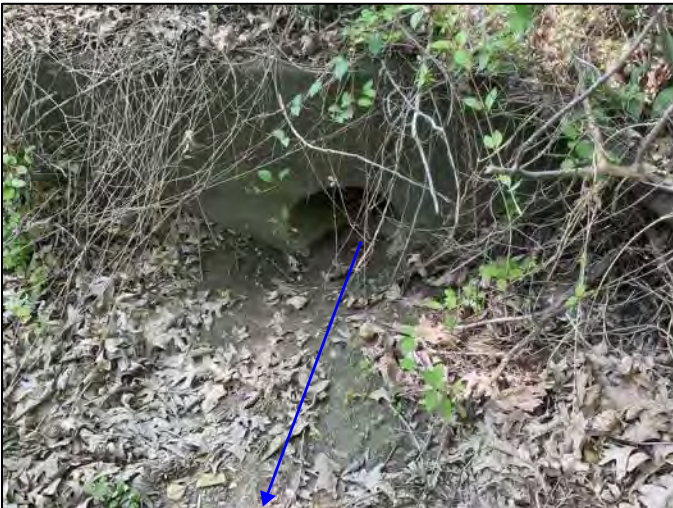
Photo 3. Outlet of CLV-67648 with UNT 3 to Beech Creek, facing upstream, viewing south, 5/13/2022
