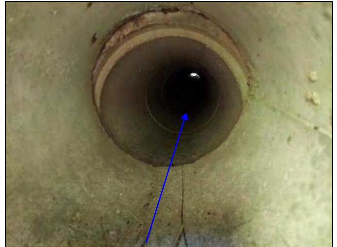
Photo 6. Looking through CLV-67648 at inlet with UNT to Beech Creek, facing downstream, viewing north 5/13/2022
