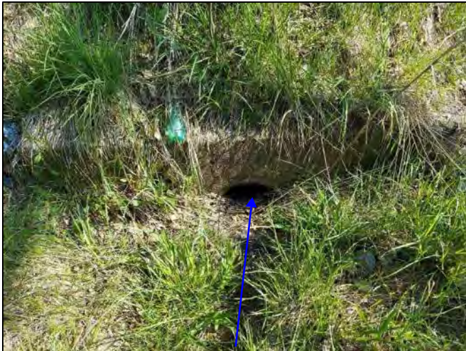
Photo 5. Inlet of CLV-67648 with UNT 3 to Beech Creek, facing downstream, viewing north, 5/13/2022
