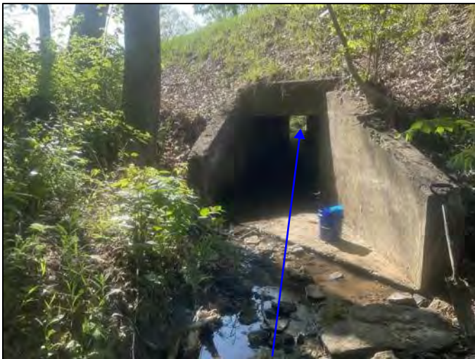
Photo 43. Inlet of culvert (CV 445-28-000.52) and UNT 1 to Beech Creek, facing downstream, viewing southeast, 5/13/2022
