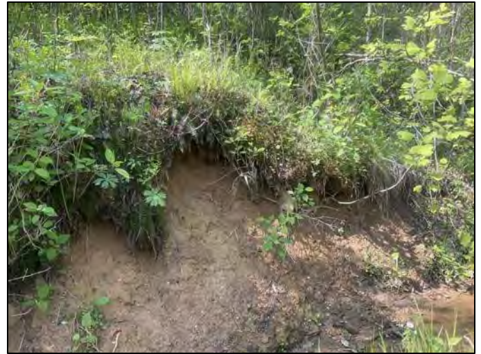
Photo 50. Eroded bank of UNT 1 to Beech Creek, viewing south, 5/13/2022
