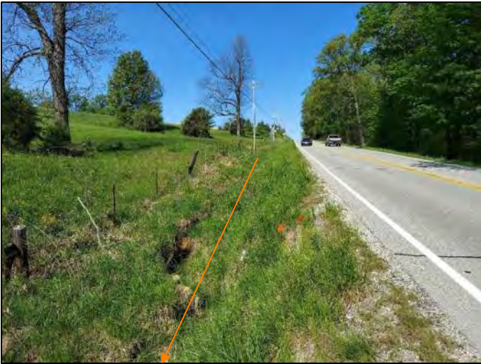
Photo 17. RSD 4 with eroded areas south of SR 445, viewing west, 5/13/2022
