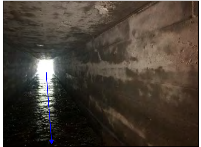
Photo 46. Looking through culvert (CV 445-28-000.52) at outlet with UNT 1 to Beech Creek, facing upstream, viewing northwest, 5/13/2022
