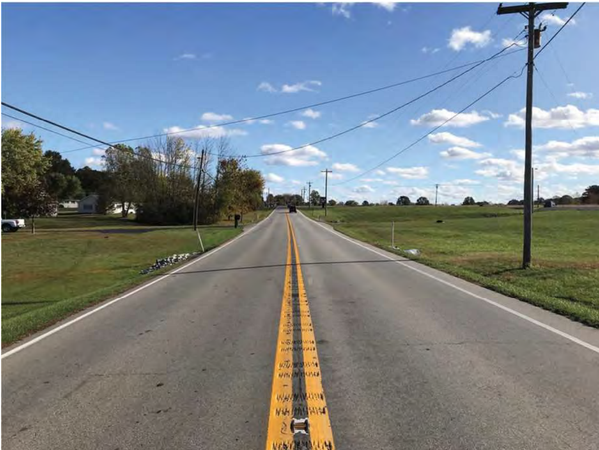
4. Looking NE from the W end of the project area on SR 56
