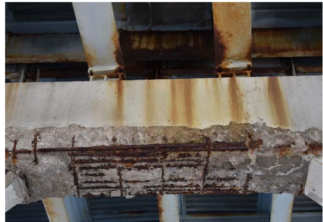
Figure 5.2.3 - Pier Cap Deterioration
