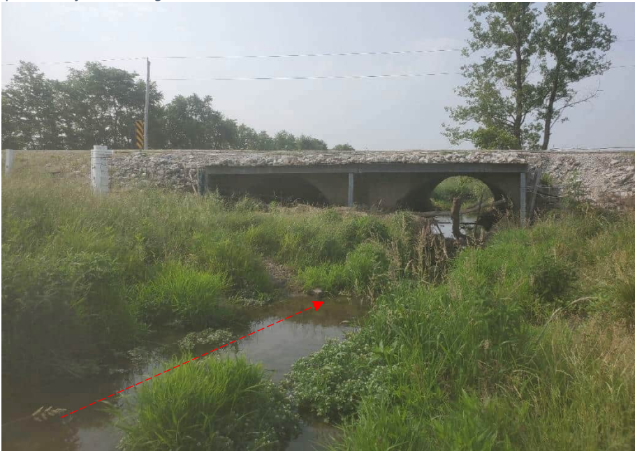
Photo 10. Facing south toward the project structure along McFarland Ditch from northwest quadrant of the investigated area.
