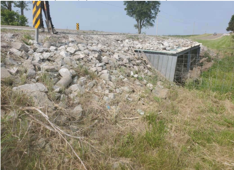
Photo 14. Facing west toward the project structure along the north side of SR 32.
