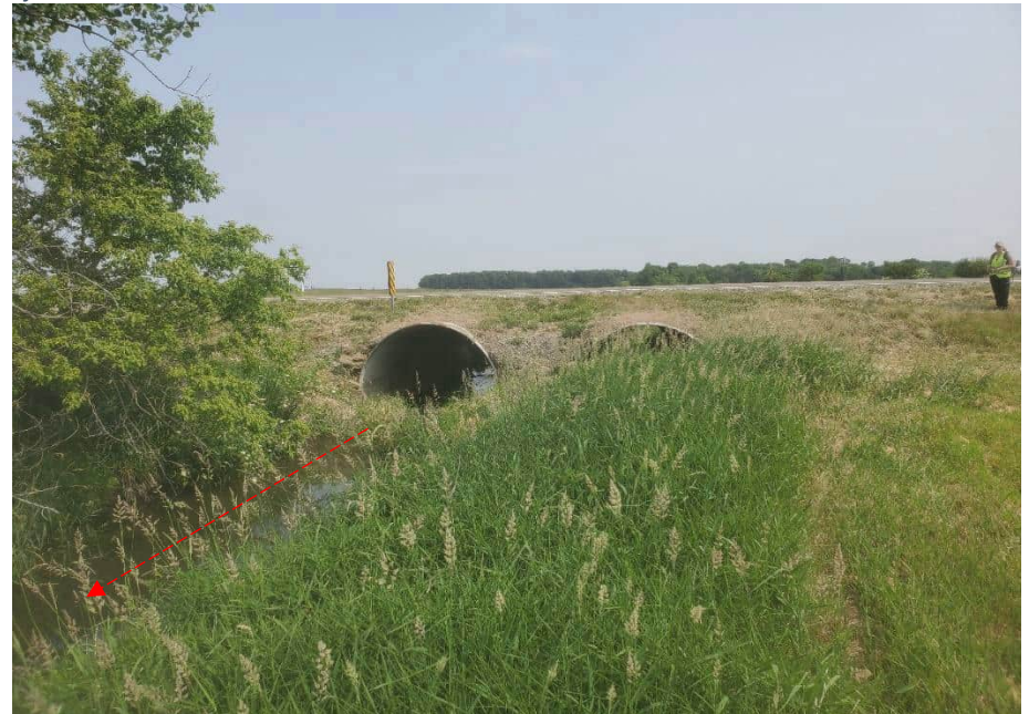
Photo 20. Facing north toward the project structure (outlet) from southeast quadrant of the investigated area.
