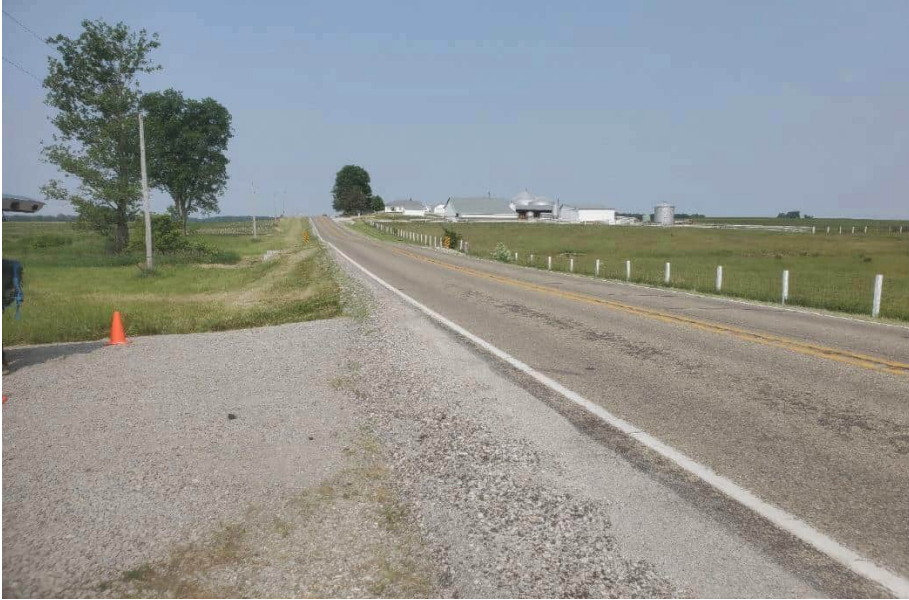
Photo 29. Facing west toward the project structure along south side of SR 32 from eastern terminus of the investigated area.
