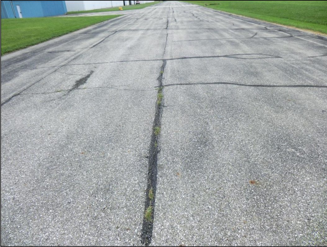
Figure 2-4. Typical Fair AC Pavement (Feature 115)
