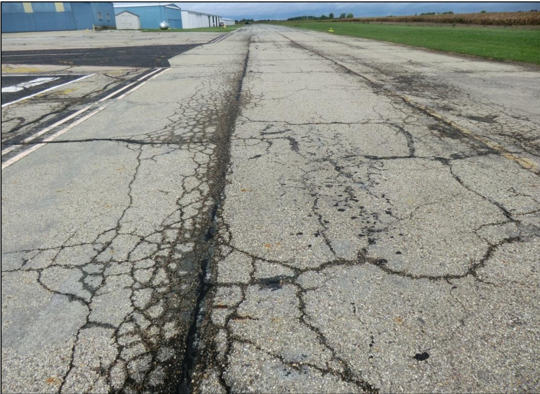
Figure 2-5. Typical Failed AC Pavement (Feature 110)
