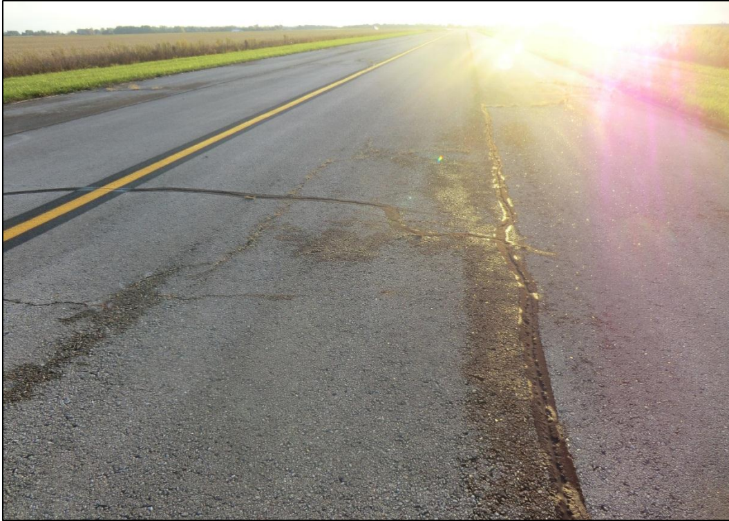
Figure 2-6. Typical Fair AC Pavement (Feature 120)
