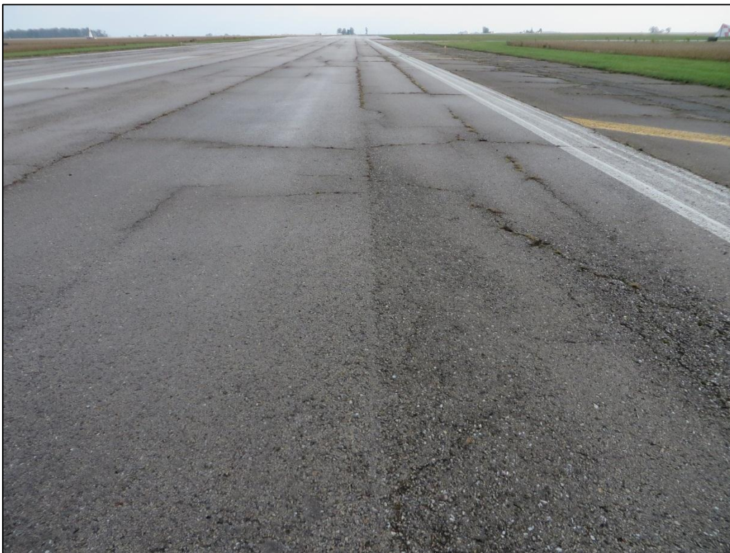
Figure 2-7. Typical Poor AC Pavement (Feature 6005)
