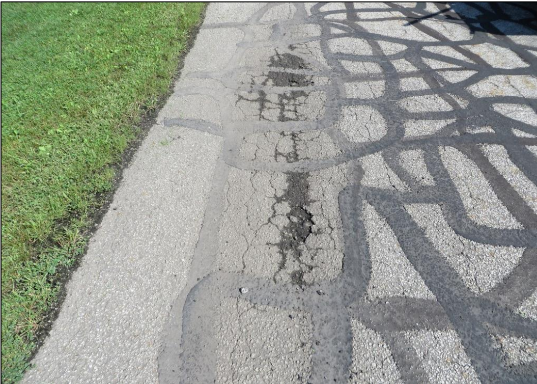
Figure 2-5. Typical Poor AC Pavement (Feature 210)
