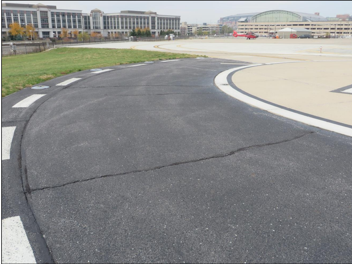
Figure 2-4. Typical Fair AC Pavement (Feature 3010)
