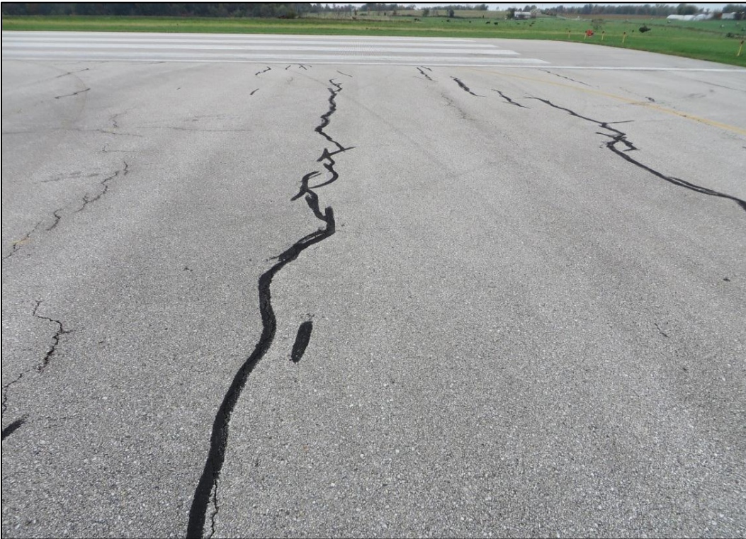
Figure 2-5. Typical Fair AC Pavement (Feature 4505)
