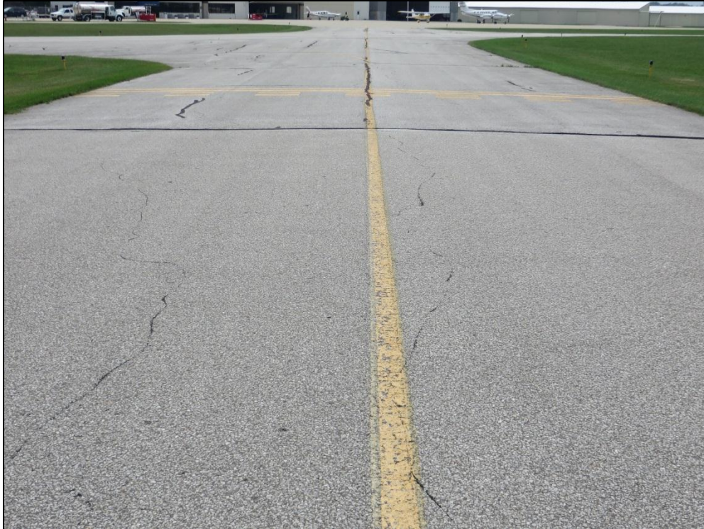
Figure 2-6. Typical Fair AC Pavement (Feature 115)
