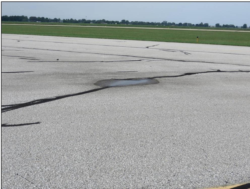
Figure 2-7. Typical Very Poor AC Pavement (Feature 120)
