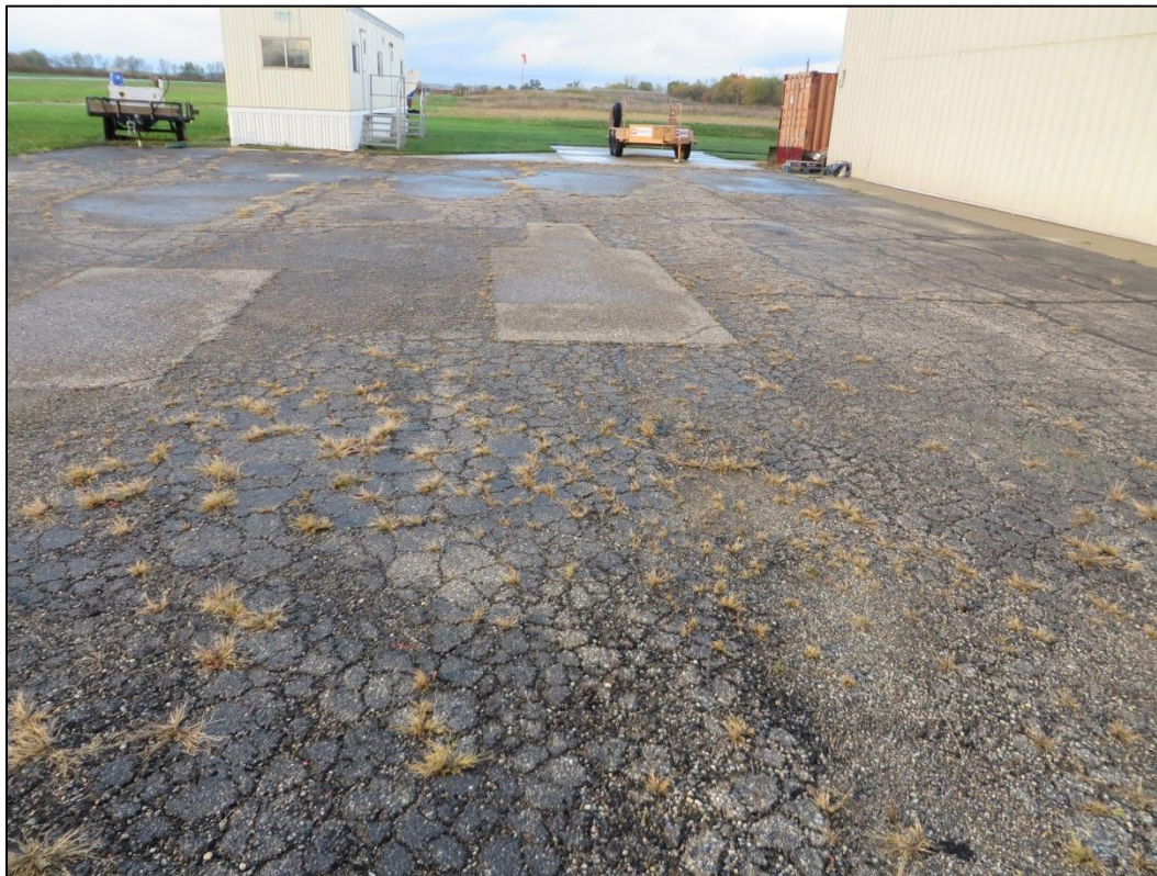
Figure 2-5. Typical Serious AC Pavement (Feature 4110)
