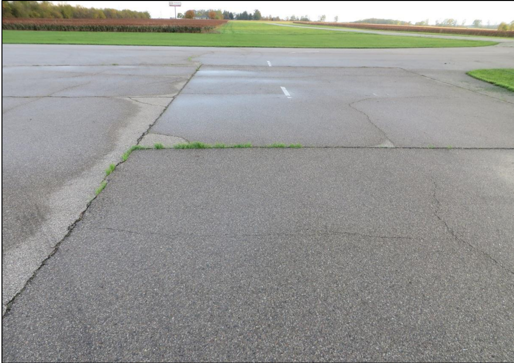
Figure 2-4. Typical Fair AC Pavement (Feature 4105)
