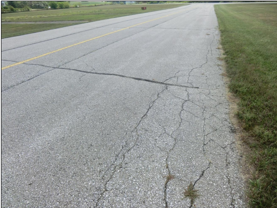
Figure 2-6. Typical Poor AC Pavement (Feature 505)
