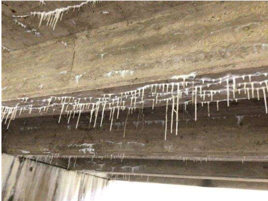
PHOTO 17 Condition Description Span f
