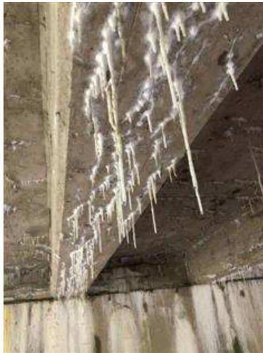
PHOTO 22 Condition Description Activity growing efflorescence on beams in span f
