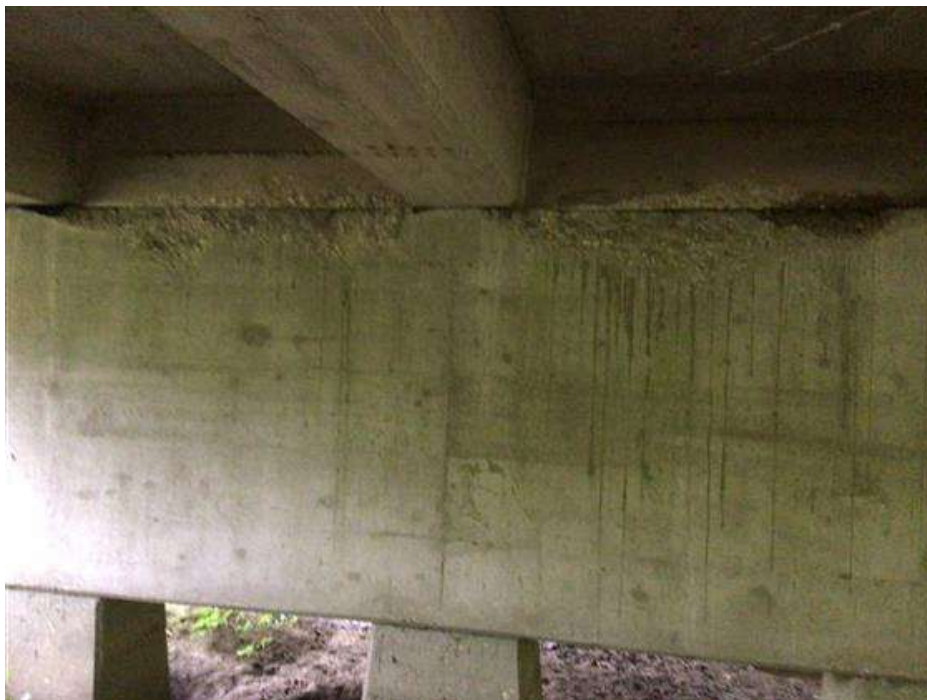
PHOTO 14 Condition Description Spalling on pier 4
