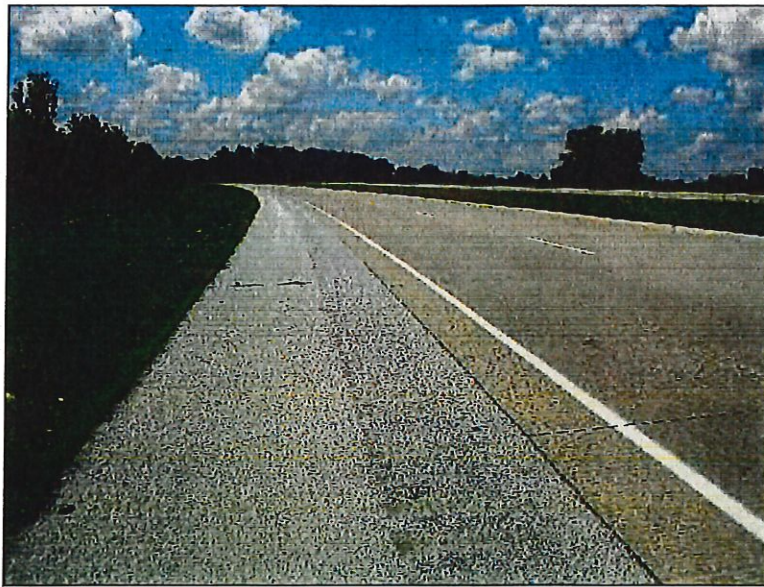
14. View looking southwest, from the western project study limits, at U.S. 24 eastbound.
