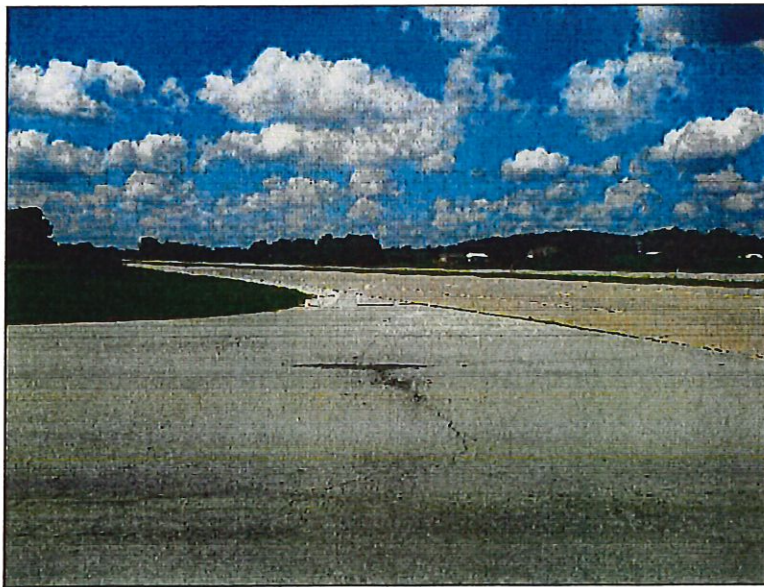
10. View from the intersection of U.S. 24 and Cement Avenue, looking west, at U.S. 24 right-of-way.
