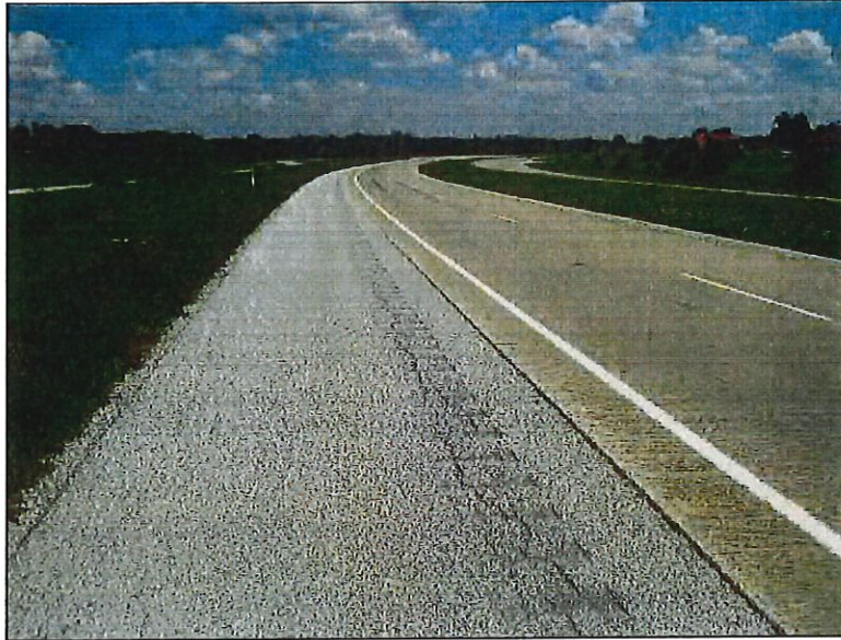
15. View from the southern project study limits, looking south along U.S. 24 westbound.
