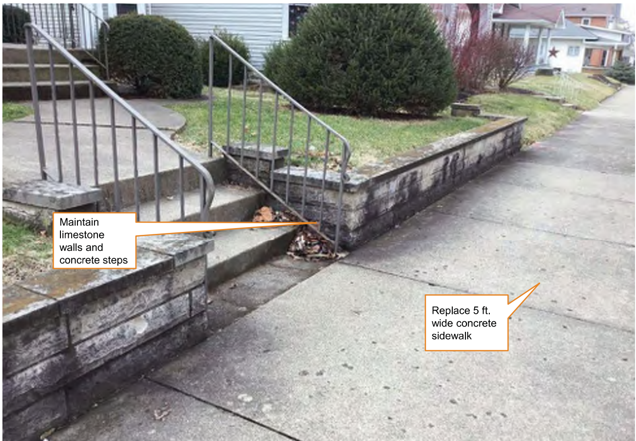
18 Looking southwest in front of "Contributing" and Non-contributing" structures within the Greensburg Eastside Residential Historic District.
