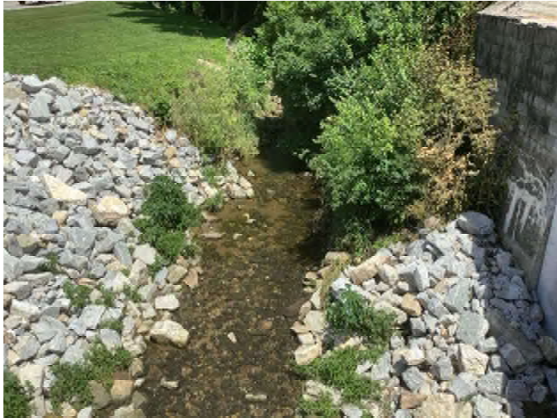
29. Facing north from Bridge No. 046-16-10454 looking at UNT 1 to Sandy Creek (locally known as Gas Creek).
