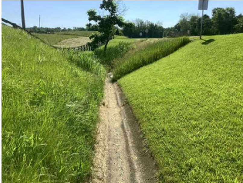
5. Facing east along the SR 46 westbound lane looking at a concrete lined ditch and at a wetland found within the project area.
