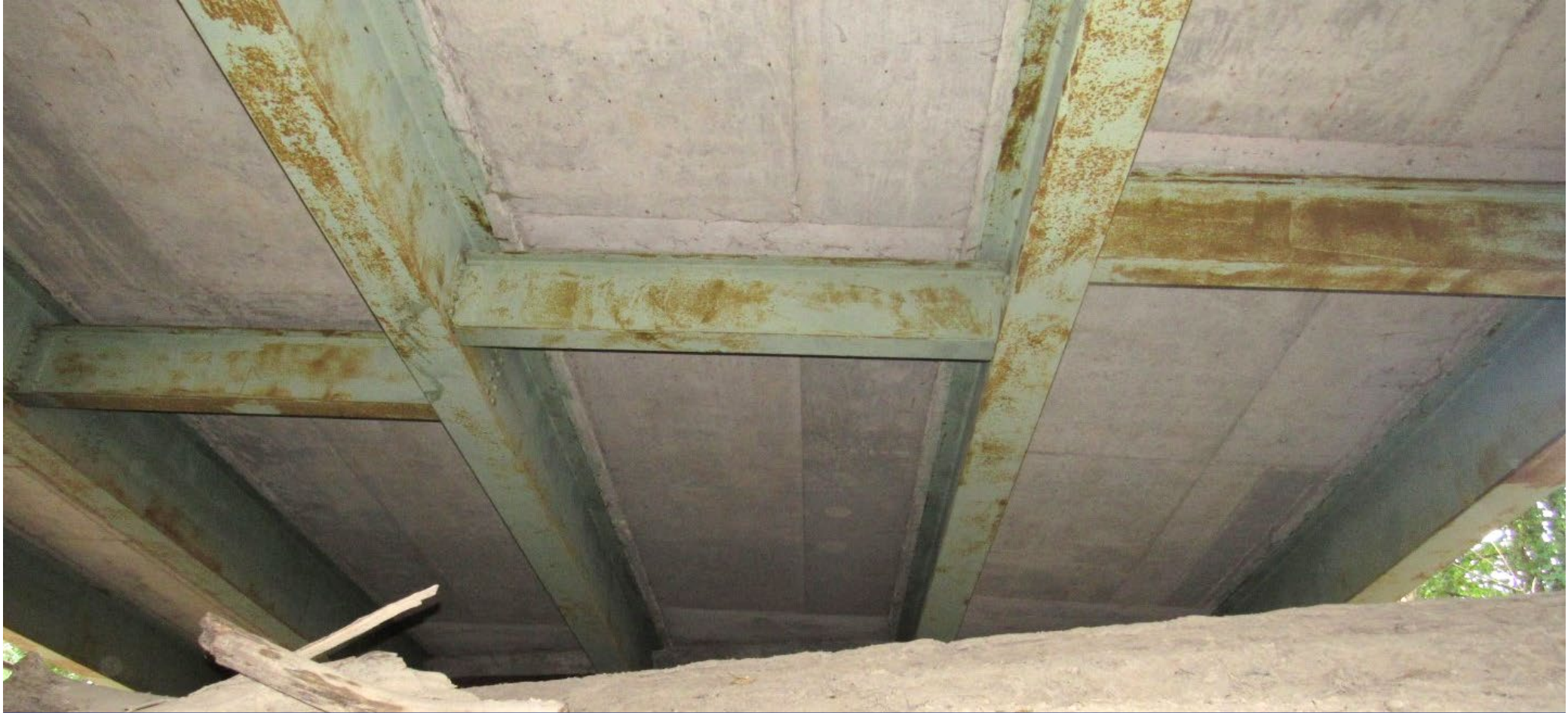
Underside of deck with medium width cracking throughout
