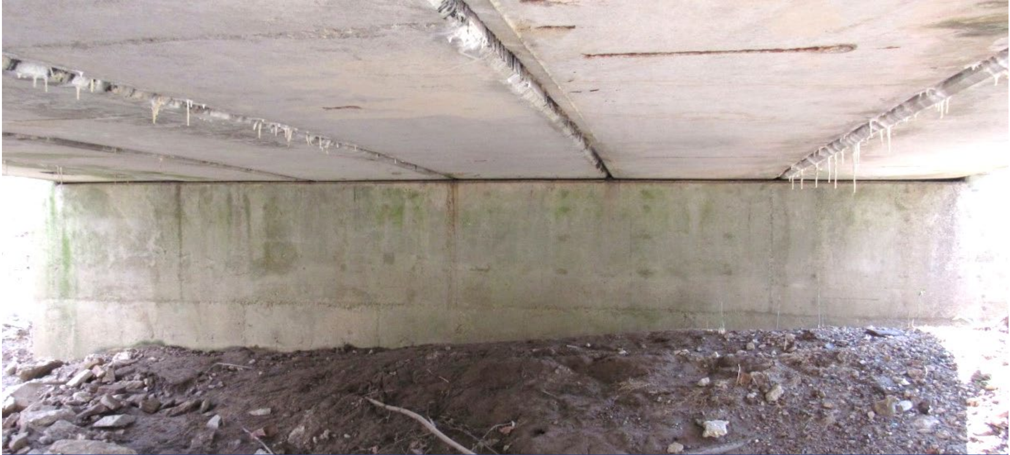
Typical minor honeycombing throughout
