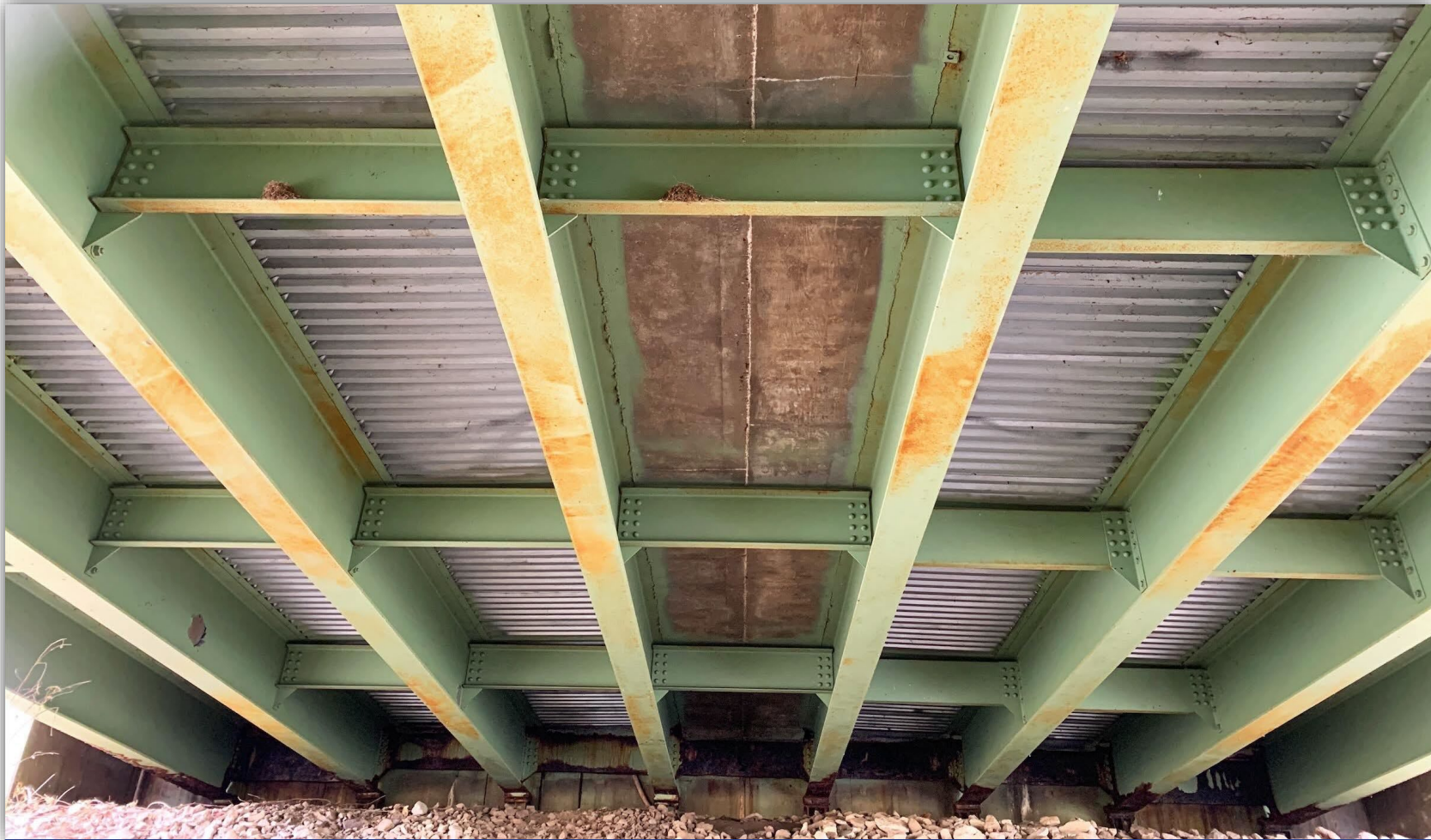
Surface rusting on bottom of flanges
