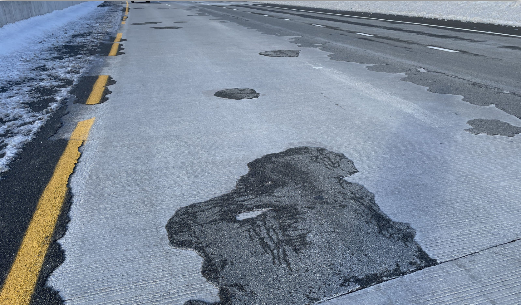
Widespread peeling, nearly 50% of bare deck exposed
