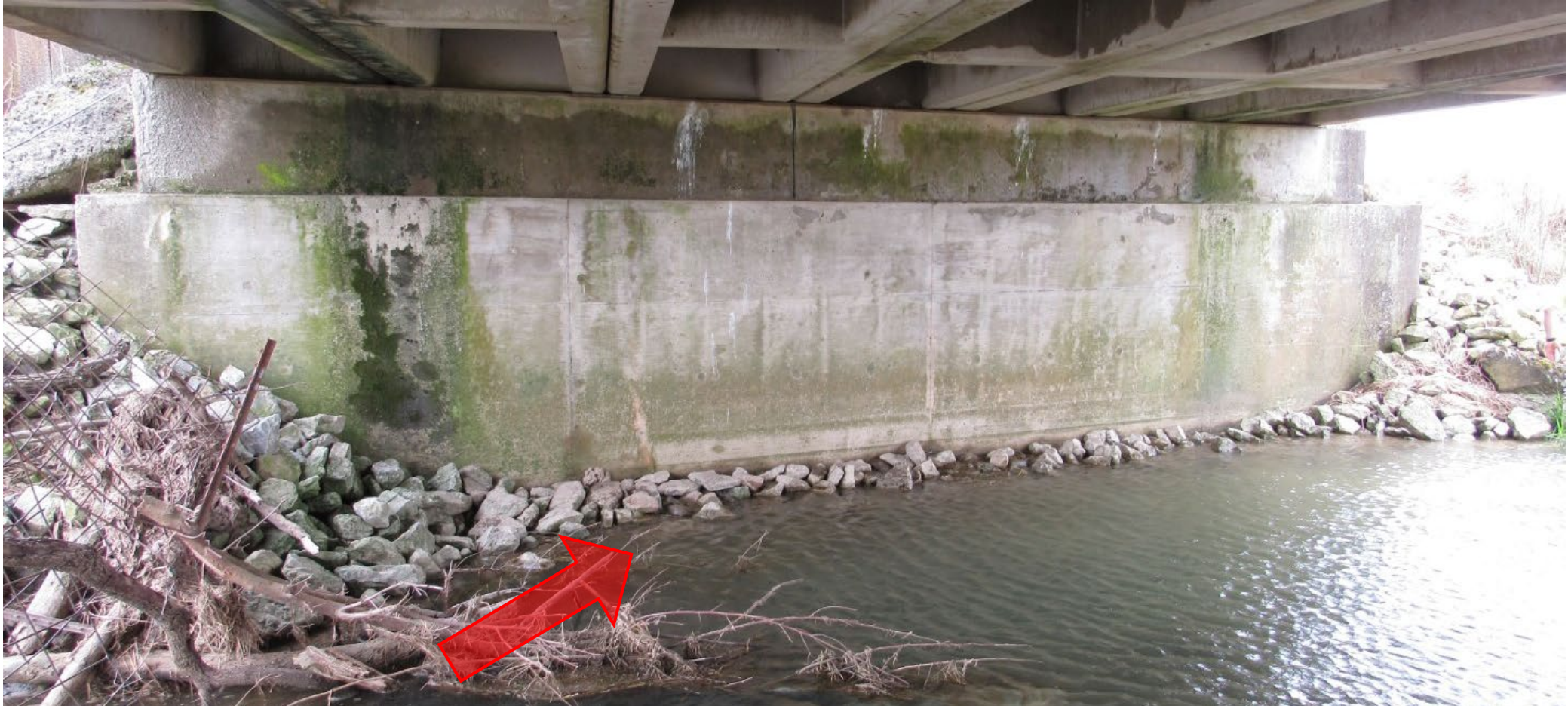
South abutment – channel impact at 20-30 degrees
