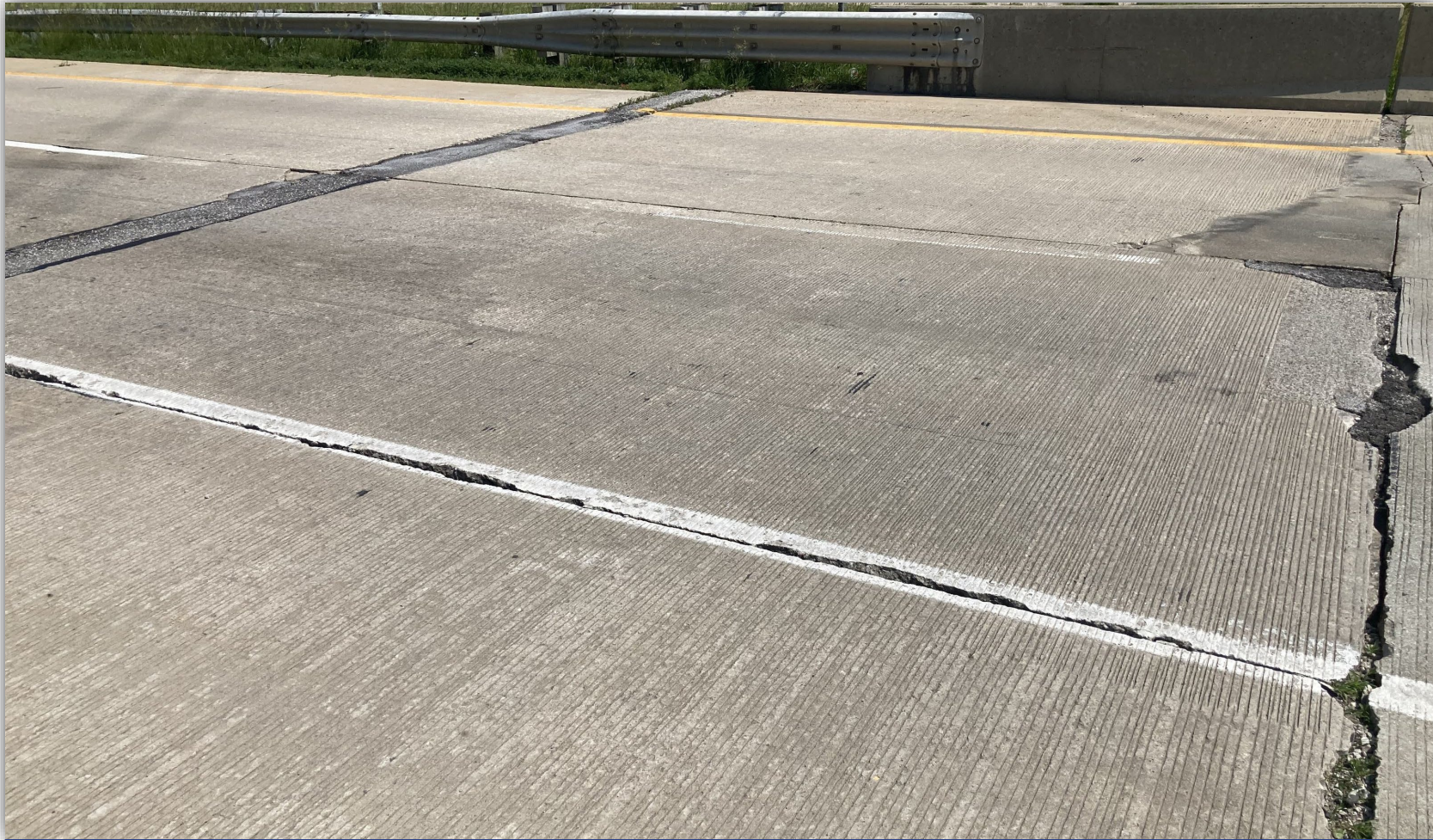
Sound patch left lane (12SF) in east approach Spalling & chipping at construction joints & bridge joint in both approaches
