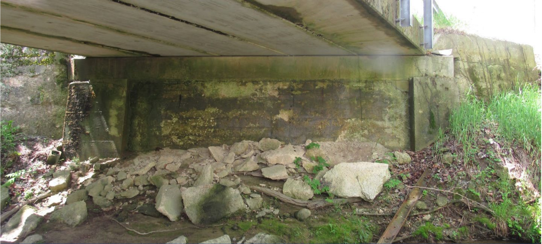
South abutment with scattered chunks of concrete and some riprap
