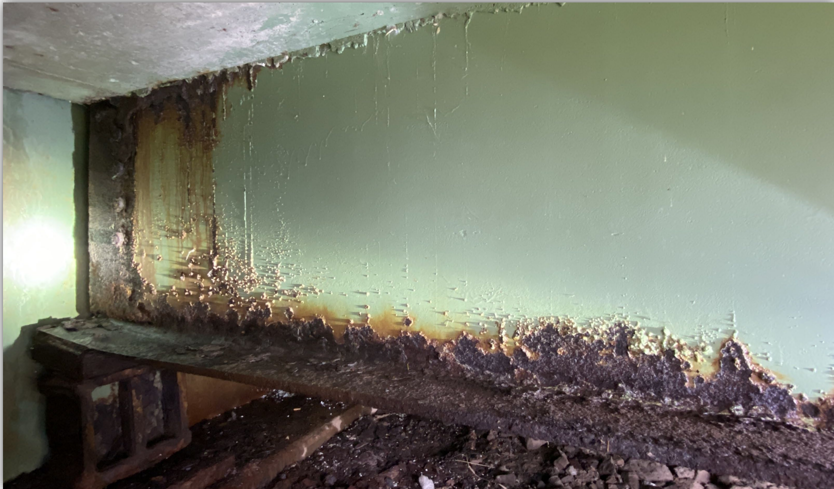
Typical corrosion at all beam ends, measurable section loss
