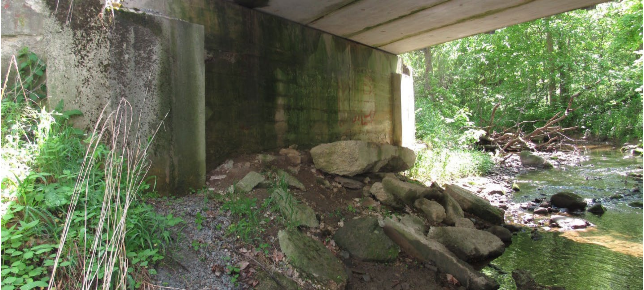
North abutment with scattered chunks of concrete and some riprap
