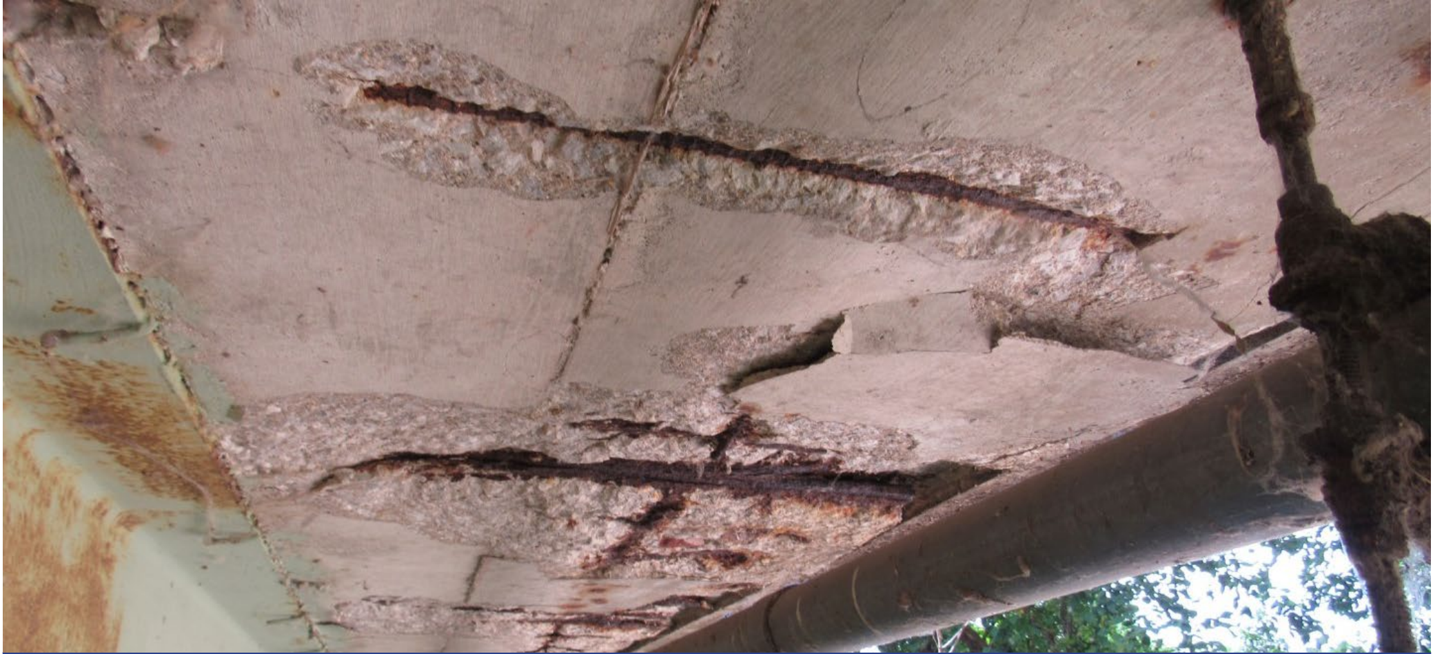
Exposed steel with minor section loss in bottom of north coping, span A
