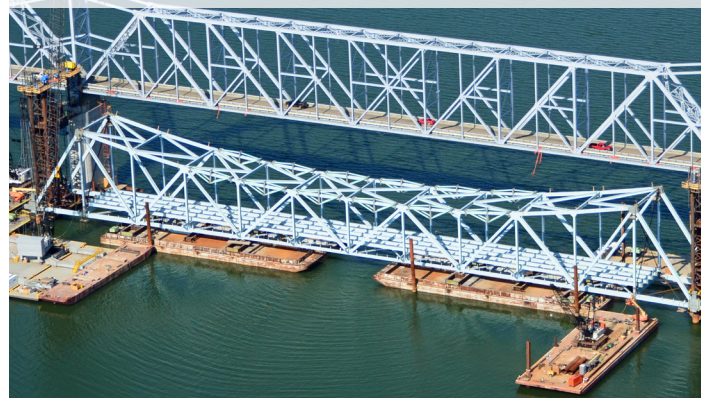
Innovative design and MOT solution to build the new Milton Madison Bridge adjacent to the existing bridge before sliding into its final alignment, eliminating one year of closure and ferry boat service.
