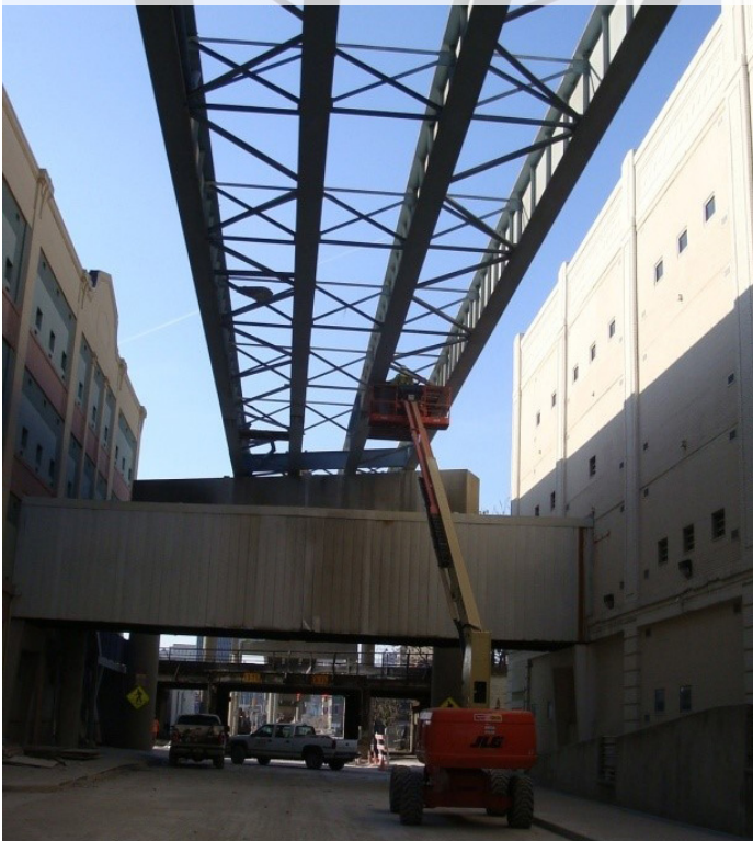
On the I-65 at Washington Street project in downtown Indianapolis, Walsh demolished the existing bridge under tight constraints in between two historic buildings.
