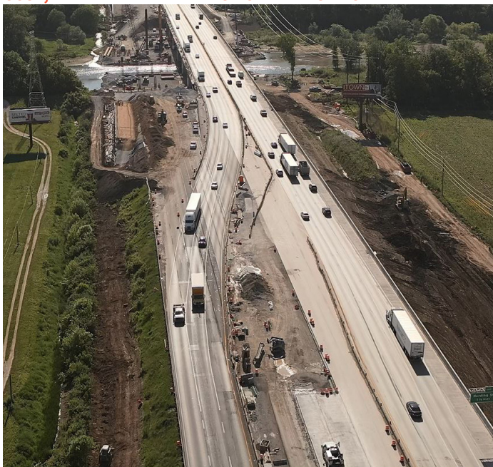
FIGURE 5.5 // ON I-69 SECTION 6.5, WALSH REDUCED 3 PHASES TO 2 BY ADJUSTING THE ALIGNMENT ON I-465. SAVED TIME, COST, AND MINIMIZED IMPACT ON THE PUBLIC.
