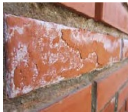
Efflorescence and spalling
