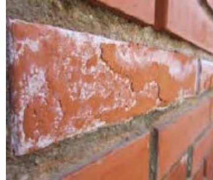
Efflorescence and spalling
