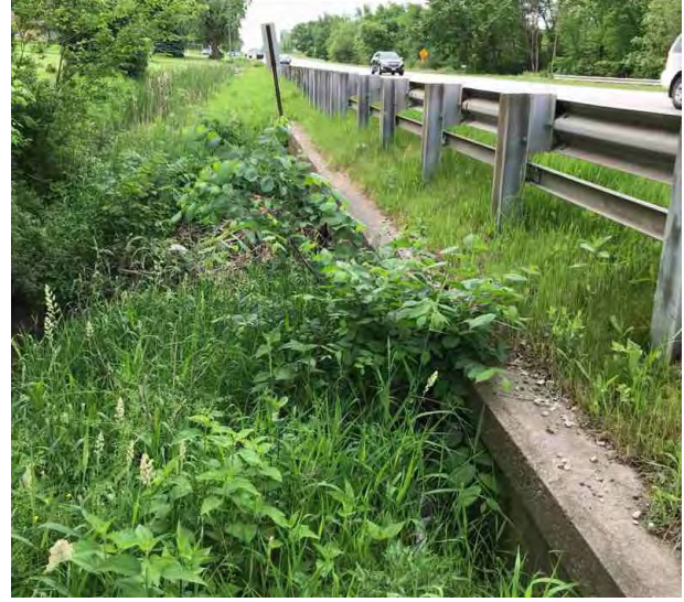
Figure 17 The eastern ditch line of US 41 facing south, as US 41 crosses the tributary of West Creek.
