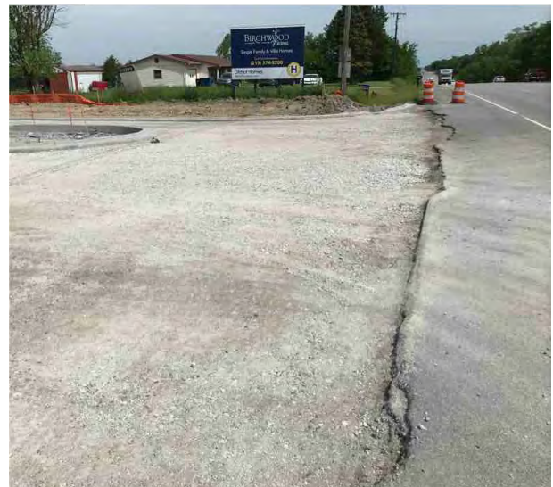
Figure 32 The western shoulder of US 41, where a new subdivision driveway is being installed, facing north.
