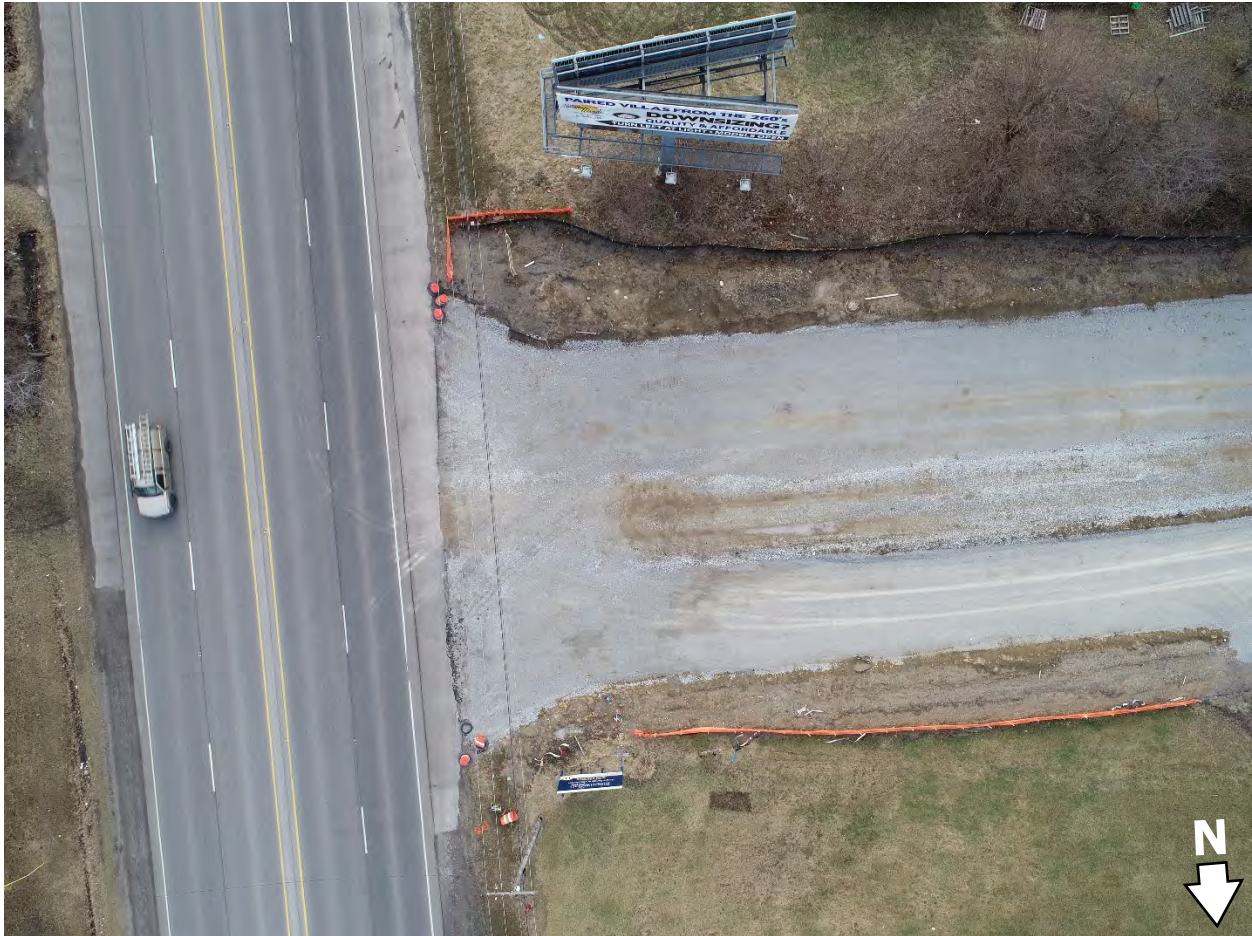
Figure 30 An aerial image of a newly constructed driveway off the western side of US 41. The image is oriented south by southwest.
