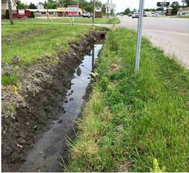
Figure 43 The western shoulder of US 41 facing north. The intersection of US 41 and W 131 st PI is pictured in the distance.
