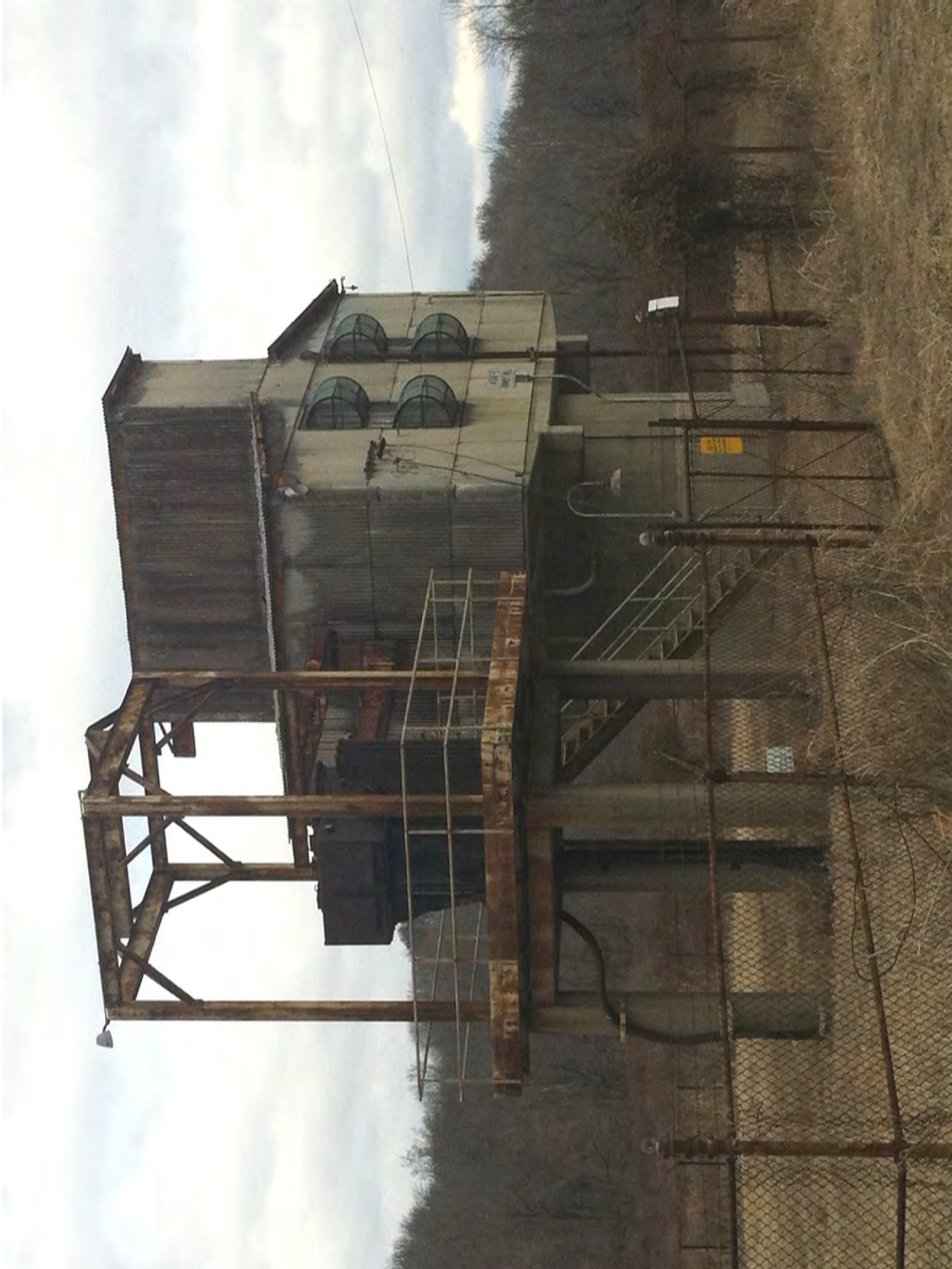
Figure 77: Collector Well CW-7
