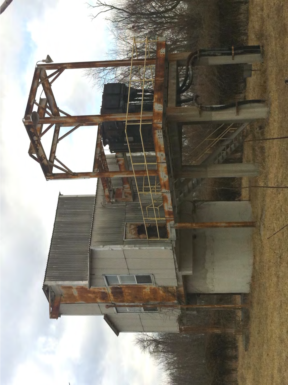
Figure 75: Collector Well CW-6
