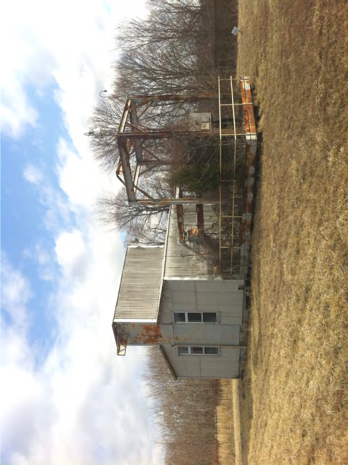
Figure 73: Collector Well CW-5
