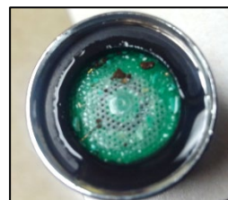
Figure 14. Photo showing a clogged faucet aerator. In this program, 7% of fixtures with aerators were above the Lead ALE. Aerators should be cleaned regularly.
