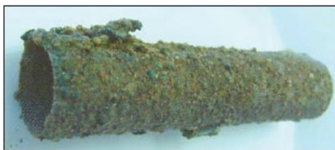
Figure 13. Photo showing a water cooler strainer clogged with Leaded debris (Elfland, 2010).
